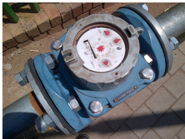
(d) Damaged meter with no glass and misaligned register
