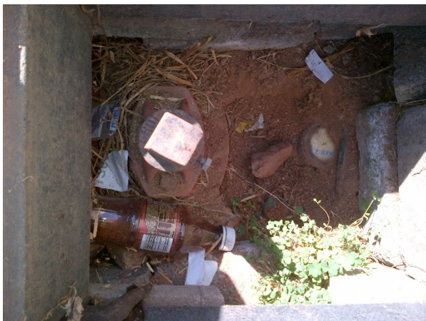
(a) Incorrectly installed meter with obstructions
