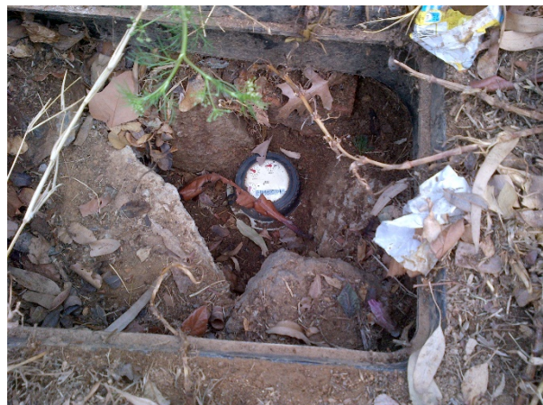
(b) Rock obstructions
