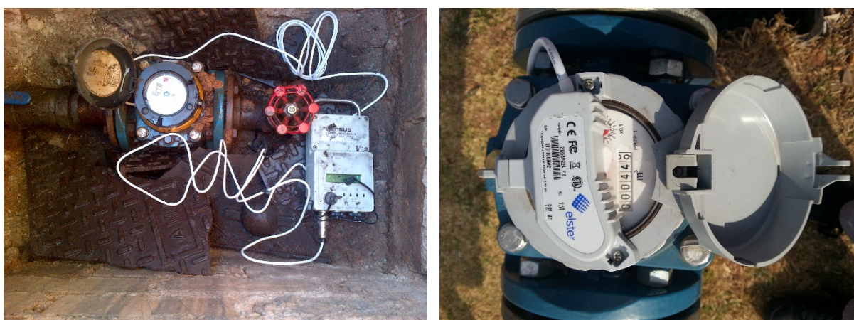
Figure 3-4: Meter Logging Setup for Large Meters
