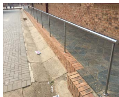
Figure 4.17. Examples of non-compliant handrails & ramps at the schools audited. (Author, 2018)
