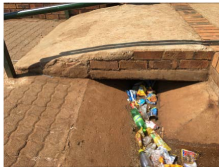
Figure 4.14. Examples of non-compliant handrails & ramps at the schools audited. (Author, 2018)
