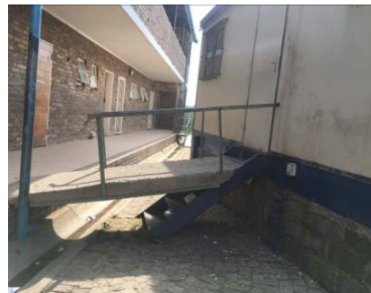
Figure 4.15. Examples of non-compliant handrails & ramps at the schools audited. (Author, 2018)
