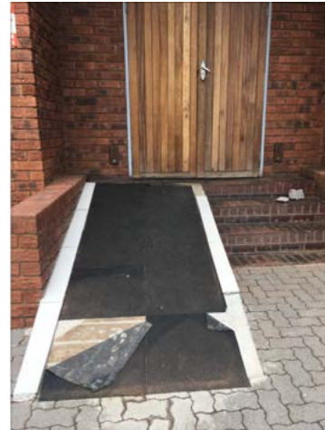
Figure 4.13. Examples of non-compliant handrails & ramps at the schools audited. (Author, 2018)
