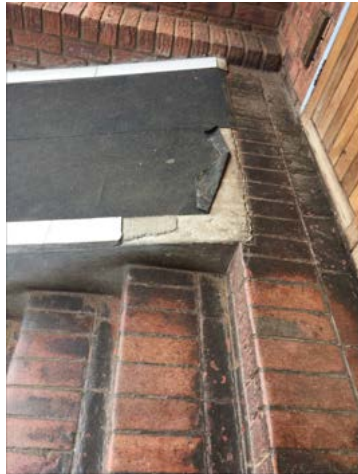
Figure 4.12. Examples of non-compliant handrails & ramps at the schools audited. (Author, 2018)
