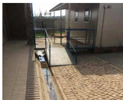
Figure 4.16. Examples of non-compliant handrails & ramps at the schools audited. (Author, 2018)
