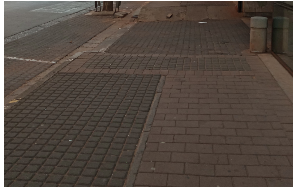
Fig 22: Colour contrast of paving along sidewalk 1b is not very sharp
