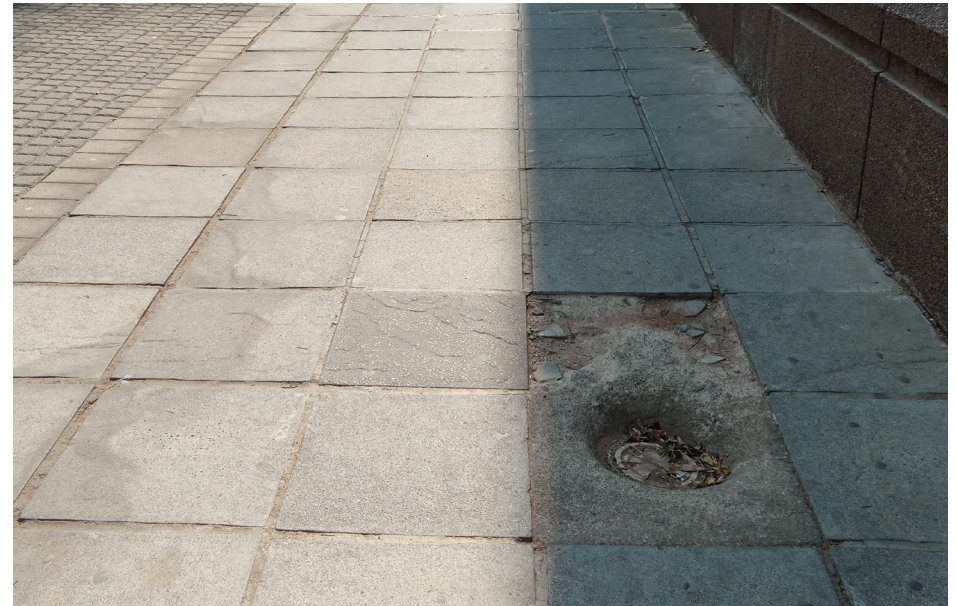
Fig 19: Missing pavers along sidewalk 4b
