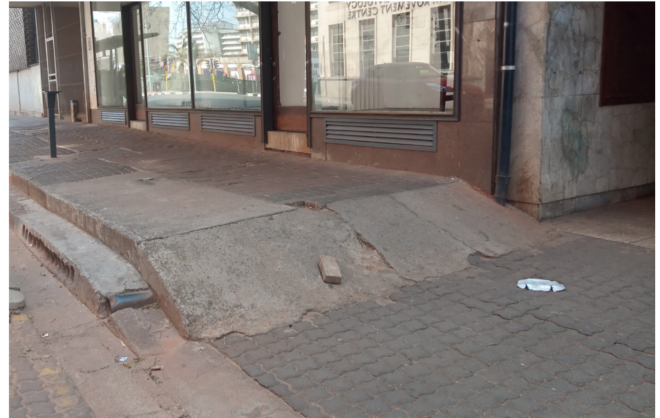
Fig 25: Steep ramp across driveway along sidewalk 1b
