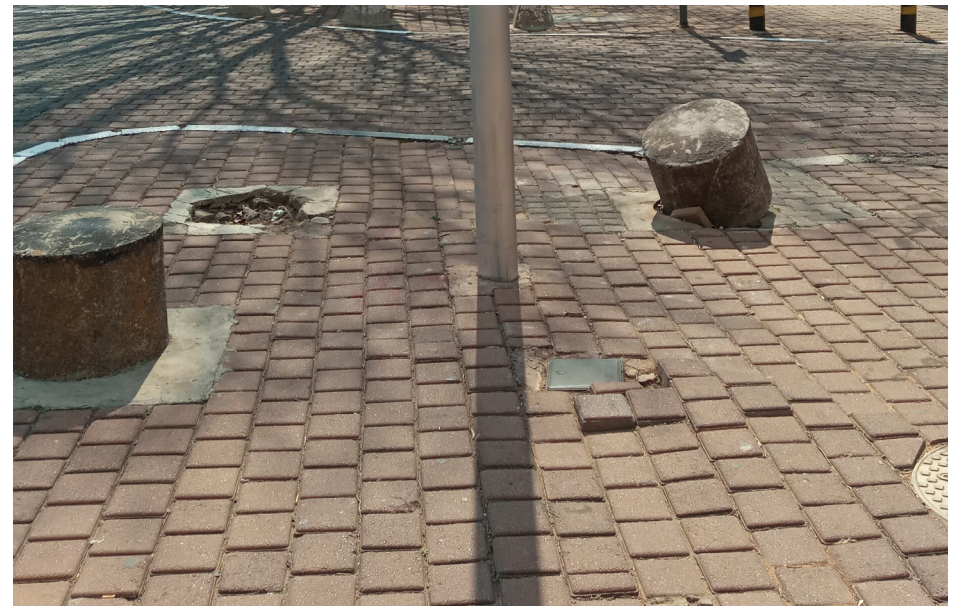
Fig 20: Uneven paving along sidewalk 4b
