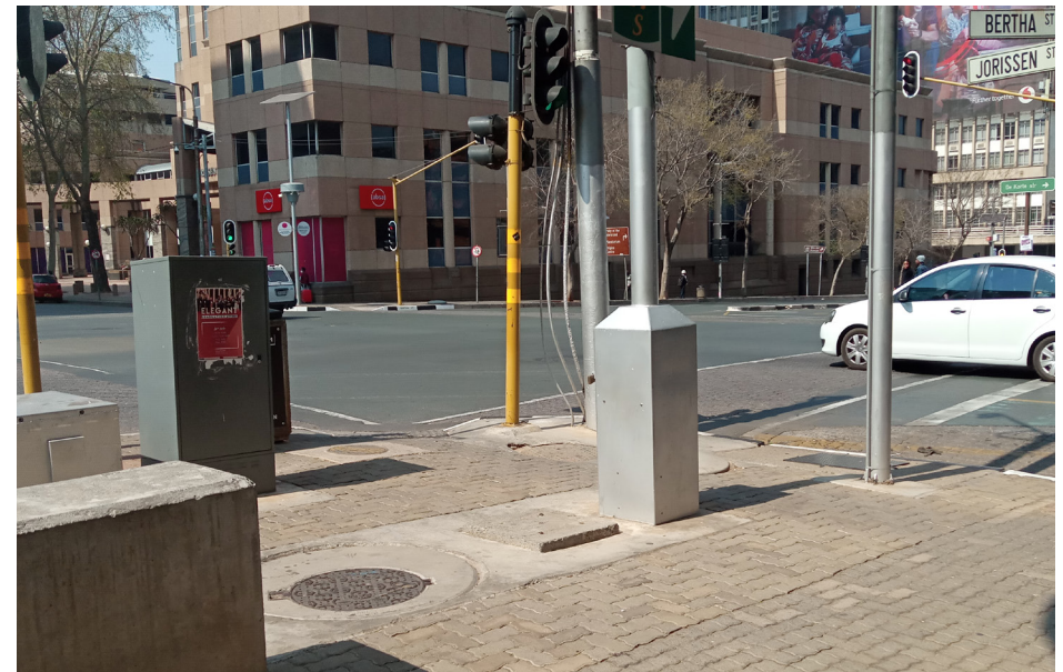
Fig 24: Numerous protrusions at the corner of sidewalks 1a and 1b
