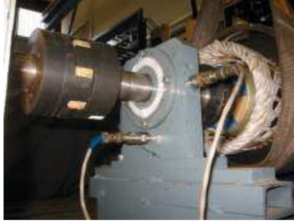
Figure 6.11: Placement of the vibration probes to measure radial and axial vibrations on the drive end bearing
