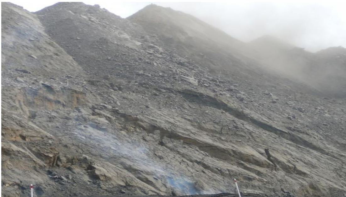
Figure 2.7: Circular failure at New Vaal Coal mine.
