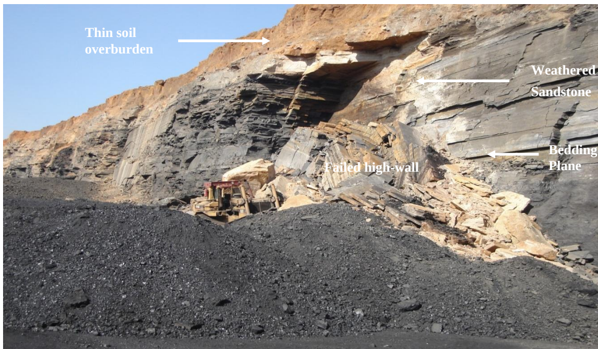
Figure 4.9: Failed high-wall at Landau open-cast mine (Landau Colliery, 2009).
