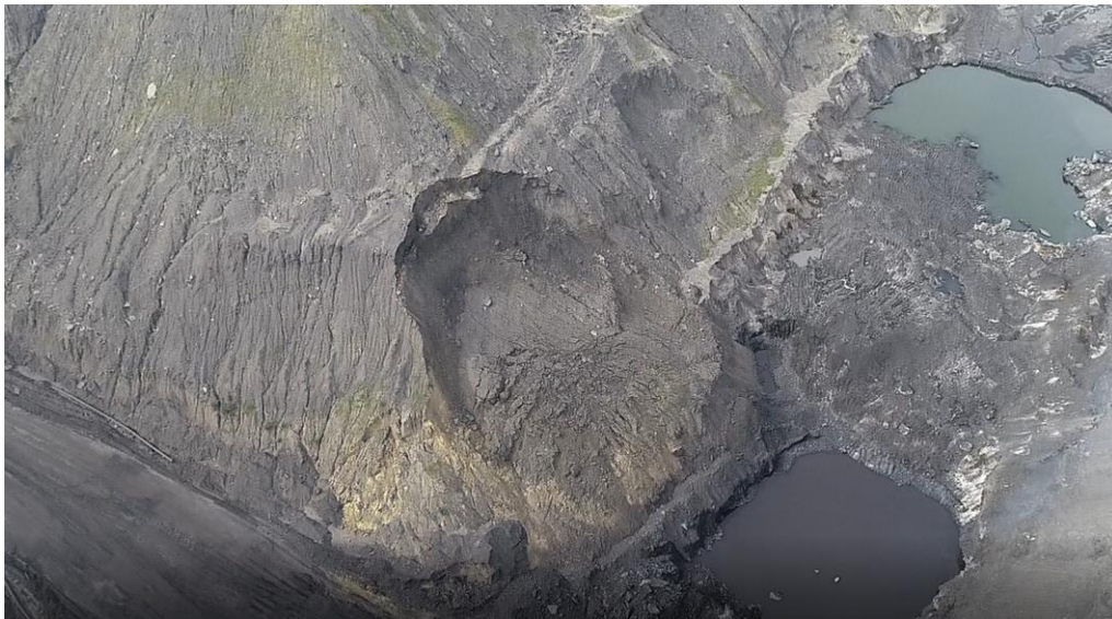
Figure 13: Ramp 20 low wall failure that occurred on 30 March 2019.
