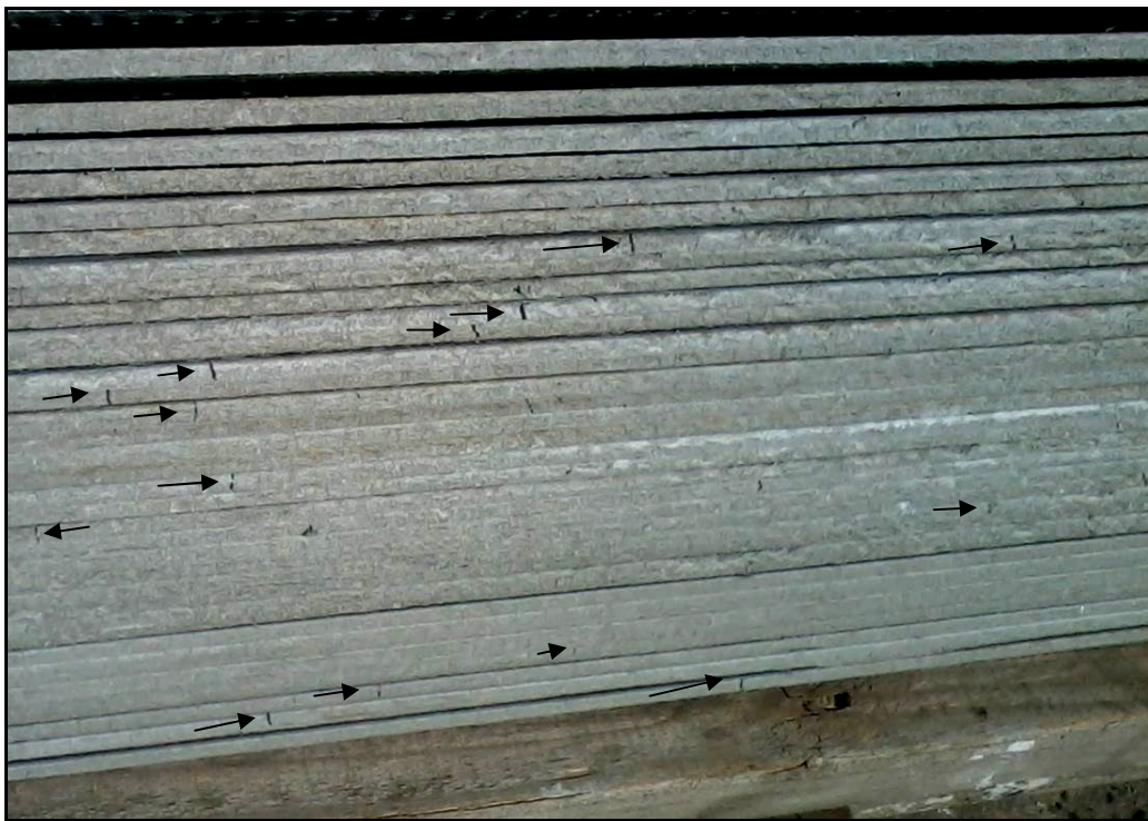
Figure 6.42: A stack of 3% kaolin, replacing cement, modified corrugated sheets that were stored indoors shrink-wrapped in plastic.
