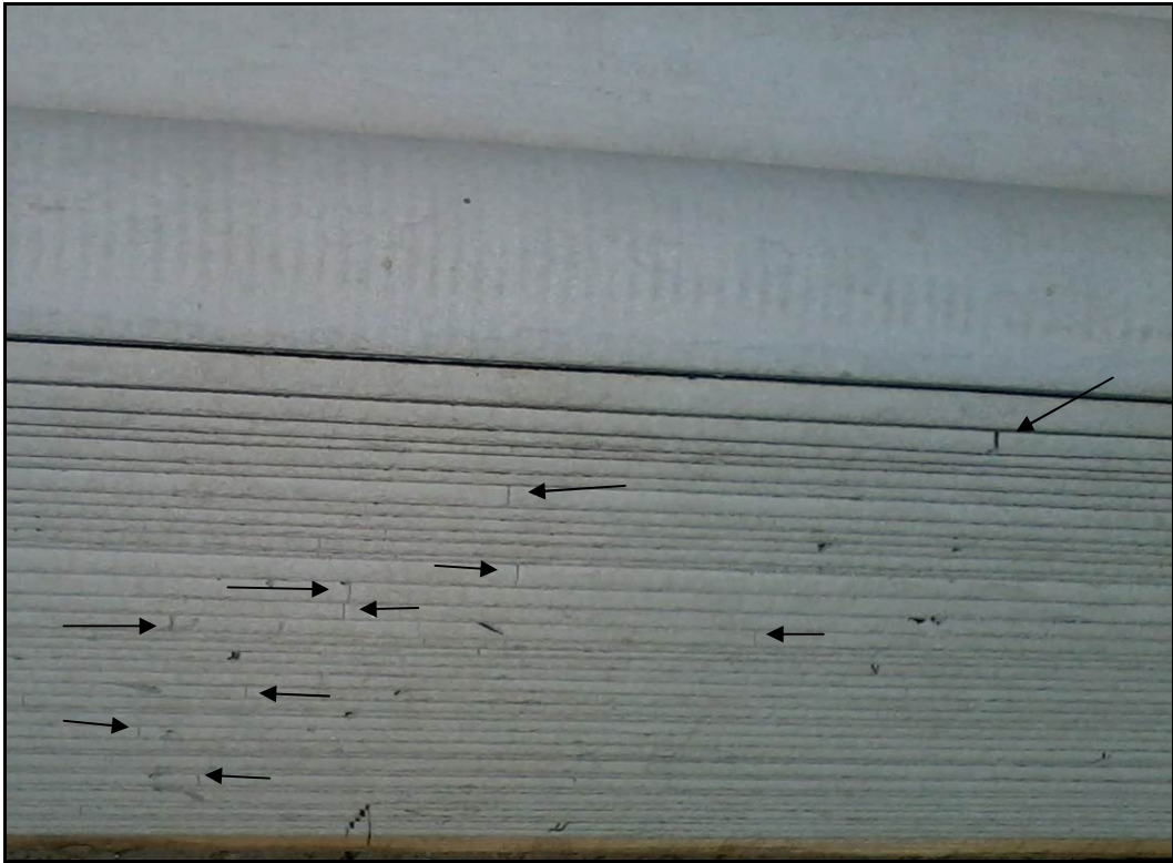
Figure 6.34: Corrugated sheets stored internally, with plastic wrapping, then cured outside without wrapping. Edge cracks appeared after 30 days curing period.
