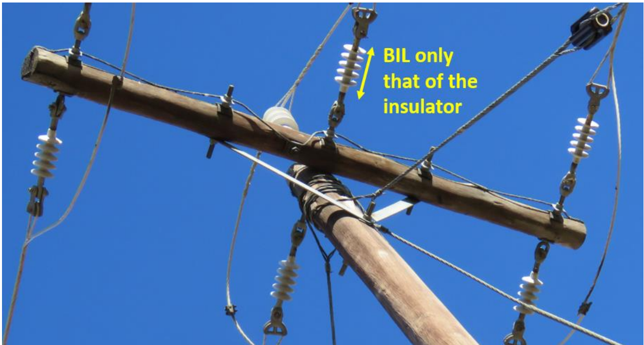
Figure 2.36 A pole-top configuration of a strain pole with stays. The BIL was limited to the insulator BIL of 150 kV. The contribution of the stay insulator to the BIL was negligible.
