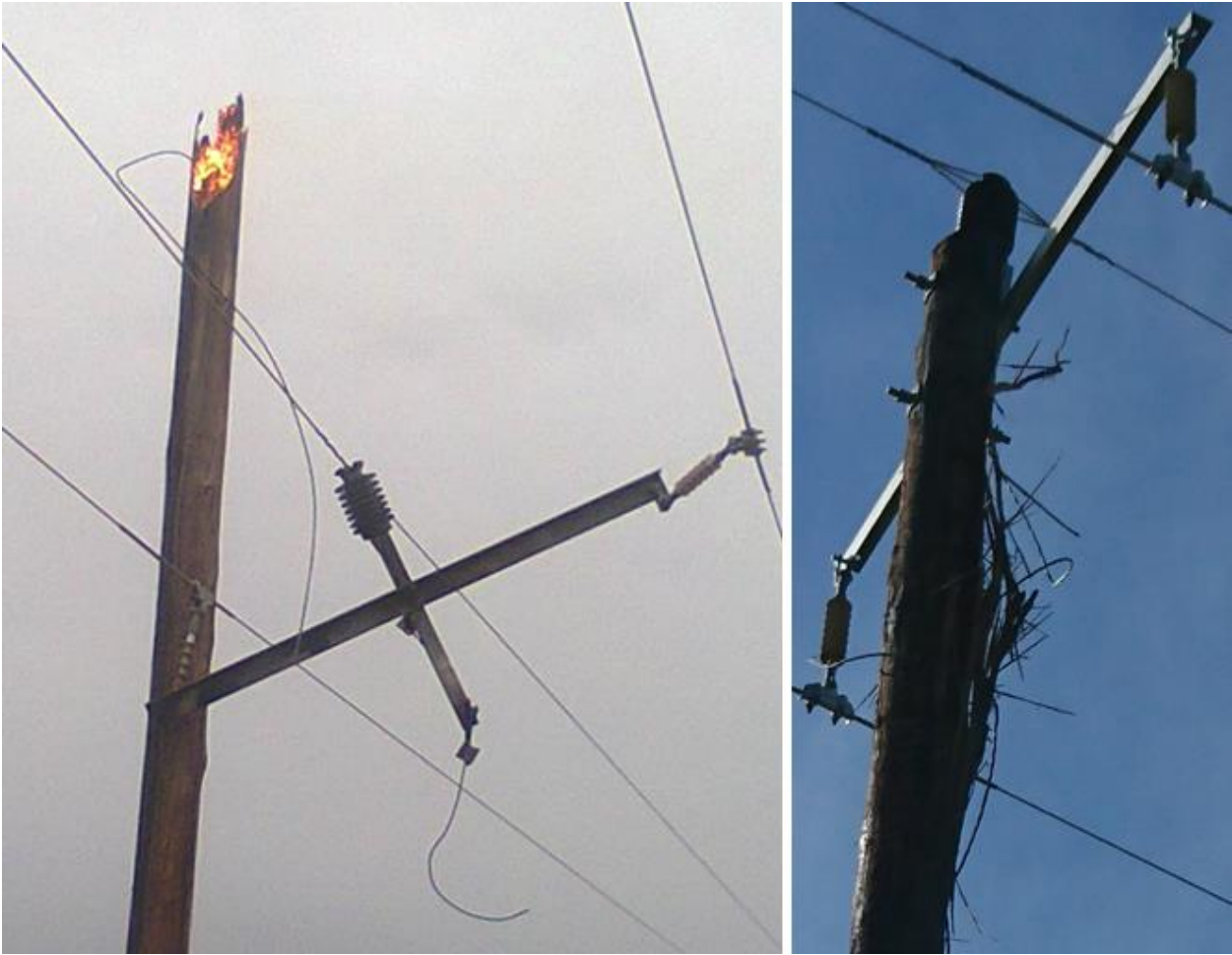
Figure 1.2 Lightning either ignites or splinters (if the lightning strike exceeds 7 kA [10]) the wood. The insulators of the charcoaled pole were tested to be in perfect order.
