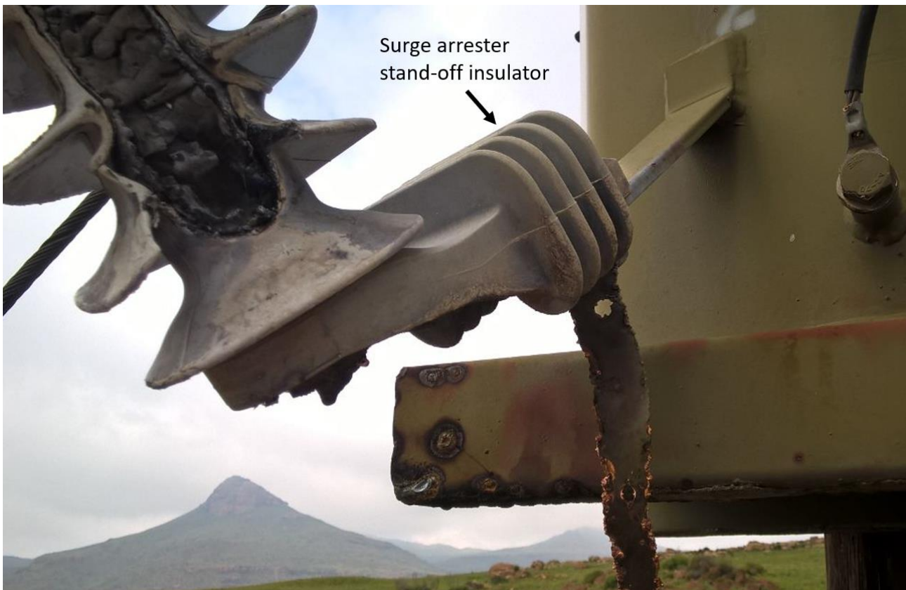
Figure 4.5 A surge arrester with a failed ground lead disconnecter. The surge arrester stand-off insulator had a very short creepage distance and the power frequency insulation was further compromised by moisture during thunderstorms.
