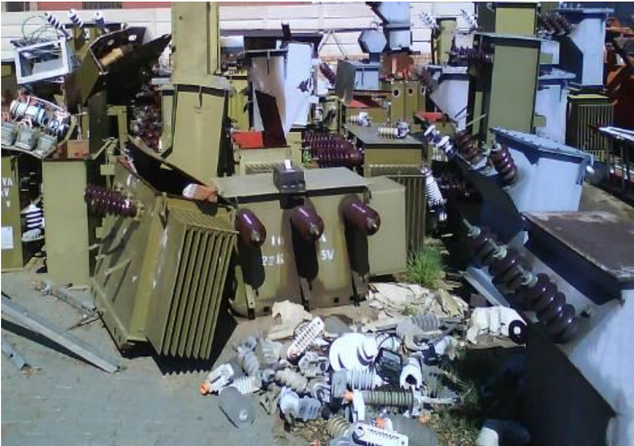
Figure 1.3 Surge arrester failures resulted in transformer failures at one of the customer Network Centres.
