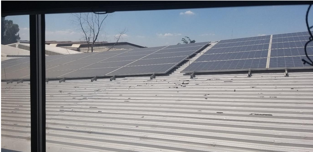
Figure 5:3 Solar roofing system on the Mpact plastic packaging factory in Wadeville, Germiston.
