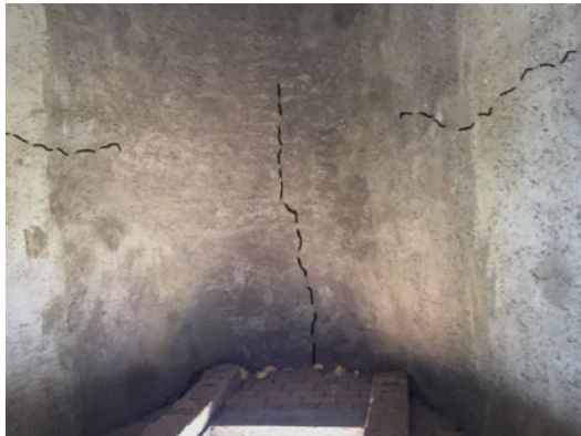
(a) Internal cracks (traced for clarity)
