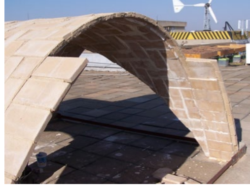
(b) Local damage at the free-edge
