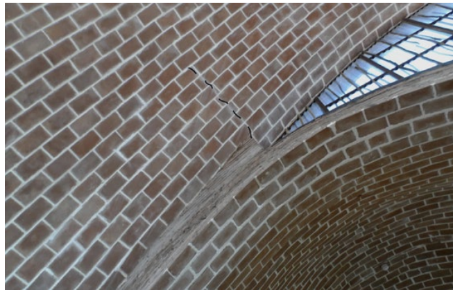
(c) Large Internal crack near shell connection/fixity
