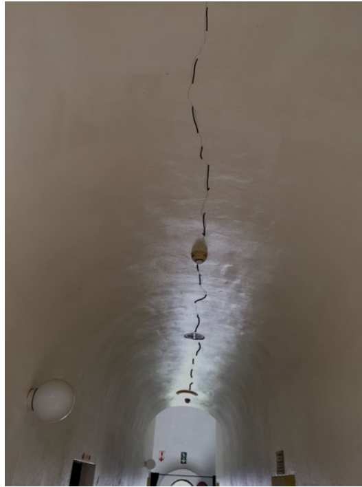
Figure 6.4 – Long apex crack in a semi-circular vault at the Sparrow Rainbow Village
