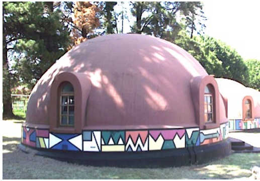
(a) Cracked dome (November, 2012)
