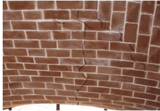
(b) Internal crack above a window frame
