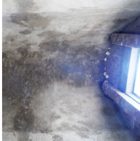
Figure 3.20 – Moisture movement through the cracks in the Wits shells
