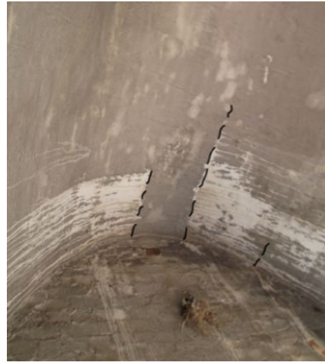
(b) Internal apex cracks (traced for clarity)
