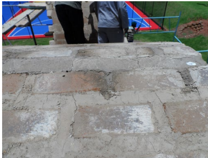
Figure 7.12 – Shrinkage cracks at the apex of the Wits vault
