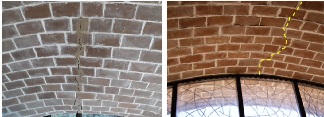
(b) Cracking above window openings
