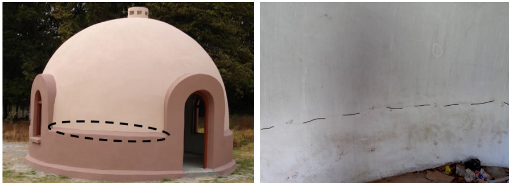
(a) Sudden change in shell thickness (b) Internal horizontal crack (traced for clarity)
