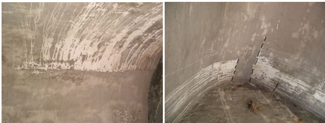
Figure 6.1 – Straight-line cracks in two of the Bapong shells (cracks traced for clarity)
