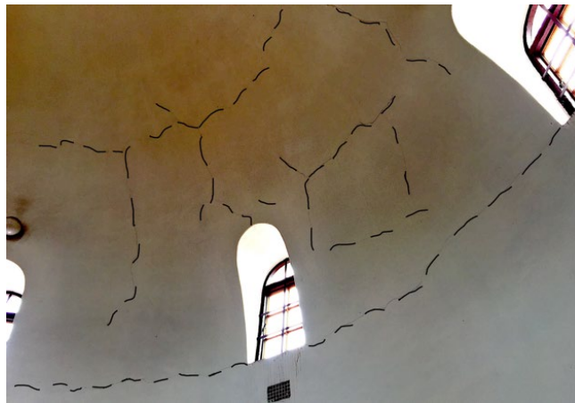
Figure 3.14 – Internal surface cracking in a CMU dome (cracks traced for clarity)
