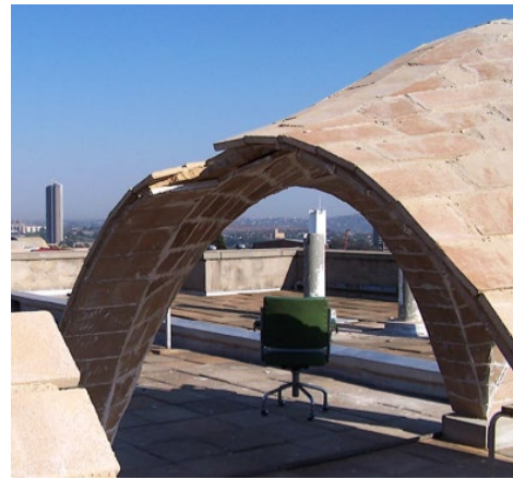
(b) Local punching damage at the free edge
