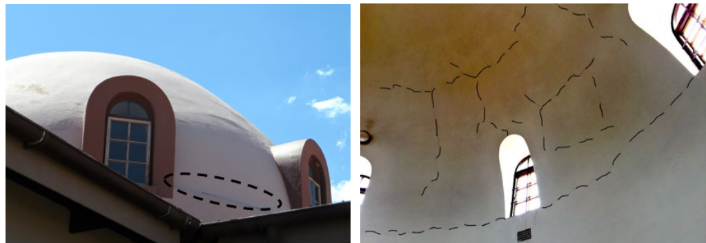
(a) Sudden change in shell thickness (b) Internal horizontal crack (traced for clarity)
