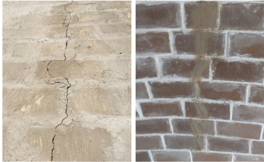
(a) External crack (blocks)
