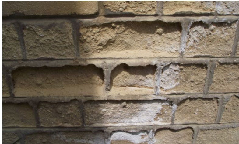
Figure 2.9 – Typical erosion pattern when mortar is stronger than the bricks, Algiers, Algeria
