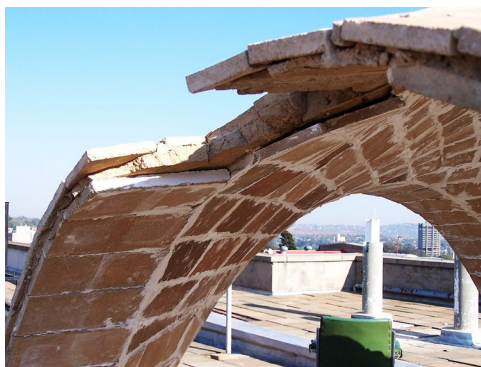
(c) Enlarged image of the punching damage
