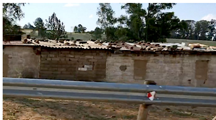
Figure 5.27 – Traditional method of preventing roof uplift (informal house adjacent to the N14 highway between Pretoria and Roodepoort)
