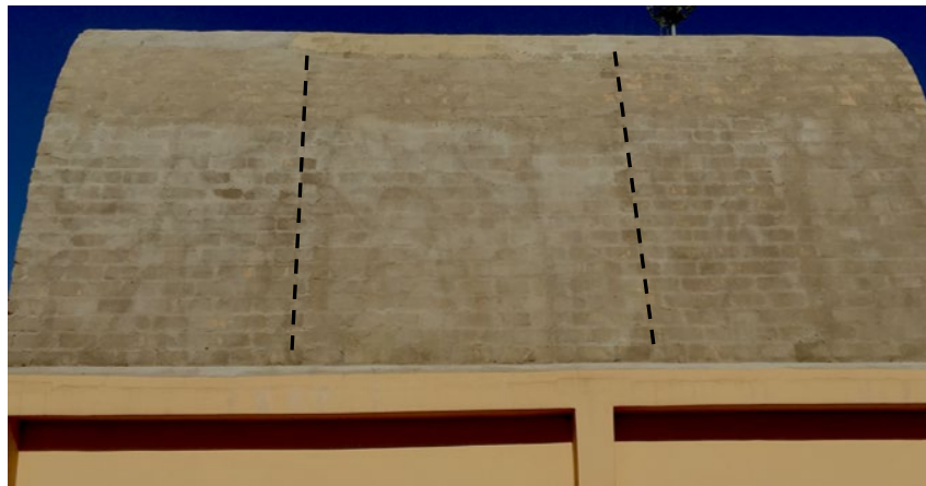
Figure 3.19 – Vertical cracks in the north-facing catenary vault (cracks traced for clarity)
