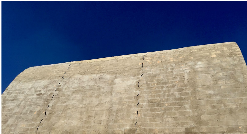
Figure 6.9 – Vertical shrinkage cracks in a CSEB vault (Bradley et al. , 2017a)
