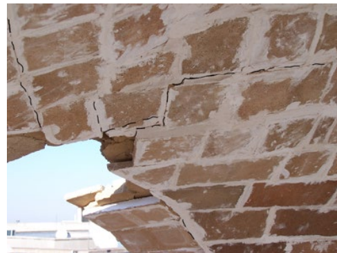
(d) Adjacent cracks (traced for clarity)
