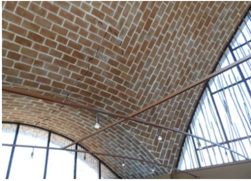
(a) Large Internal crack
