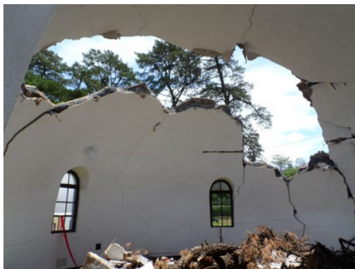
(c) Dome collapse (inside)
