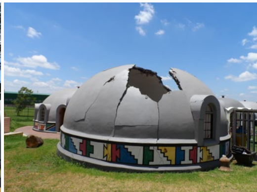
(b) Dome collapse (outside)
