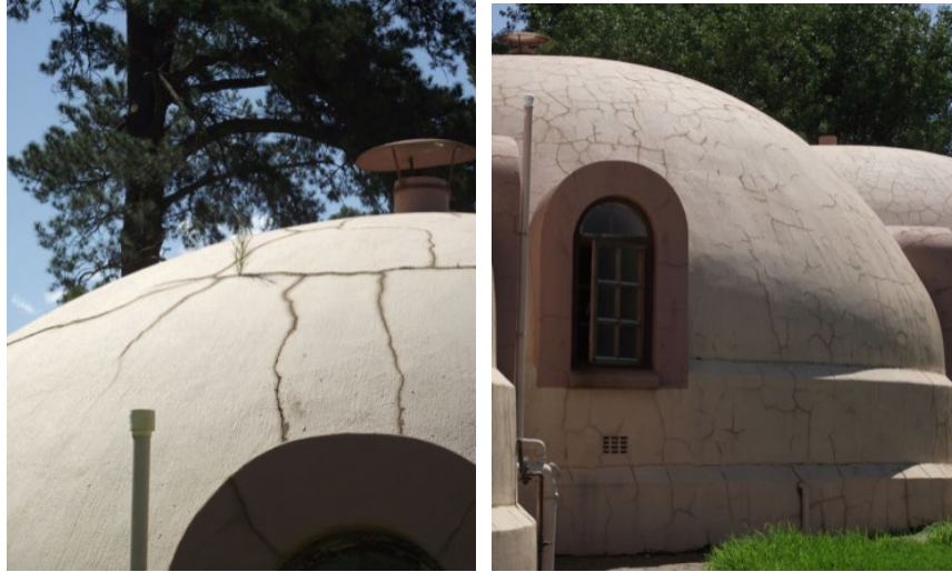
Figure 3.13 – External Surface cracking in two CMU domes
