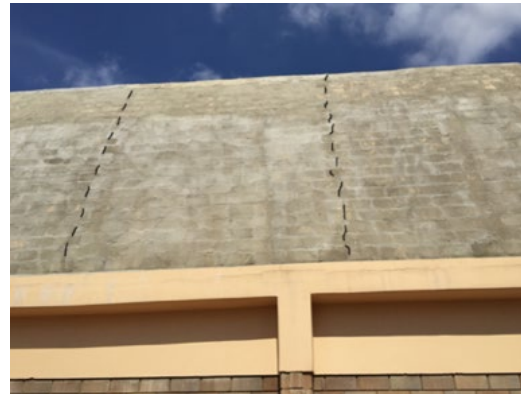
(b) External cracks (traced for clarity)
