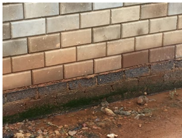
(c) Standing water, adjacent to the south-facing wall, after a thunderstorm in late 2016
