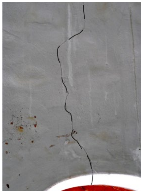
Figure 6.23 – Crack above window frame in a CSEB dome at CJC
