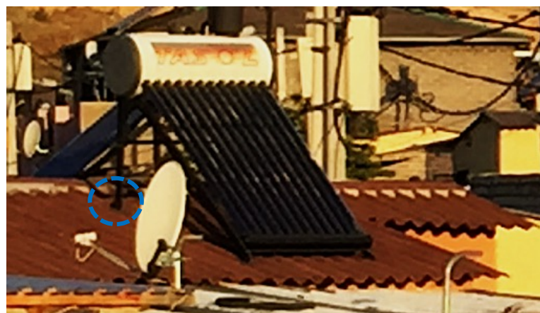
Figure 5.19 – Point loads created by a solar water heater
