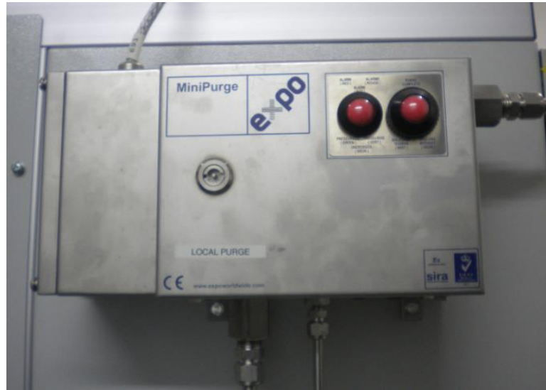
Figure 25: Expo Purge Control System
