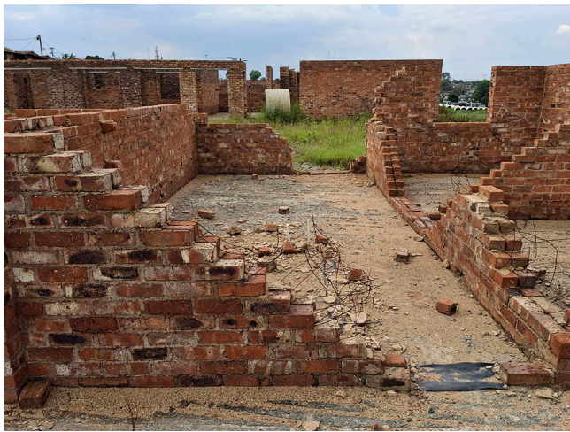
FIGURE 5B The abandoned site of the Harry Gwala housing project
