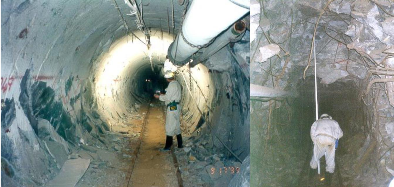
Figure 12: Damage on excavations after a seismic event (Pickering, 2013)
