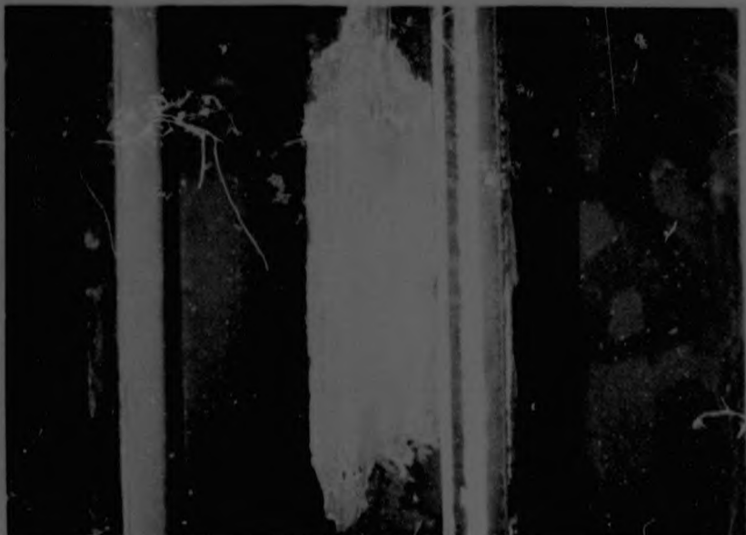
External doorframe at the J. B. Curry House indicates that the scraped surface was first stained a dark brown colour which seems to have been the standard treatment for exterior softwood application. Thereafter a white undercoat followed by green paint was applied presumably in the early years of this century. The original stain was applied in 1889.
