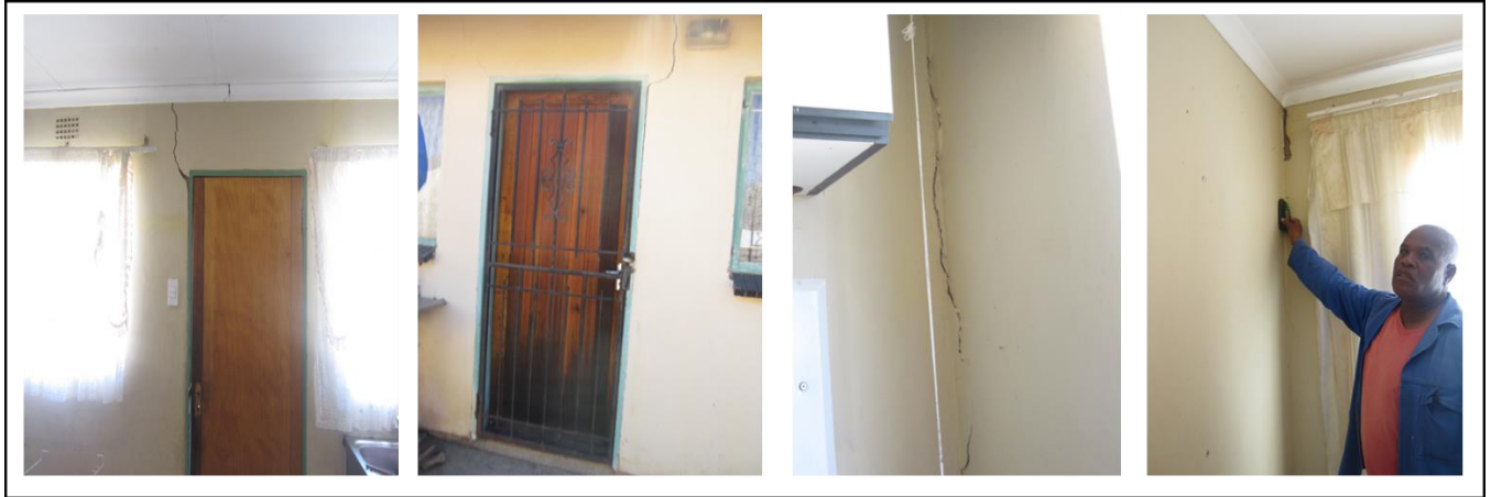
Plate 6: Some of the visible cracks in Nthate Masheane's new home in Sterkwater village
