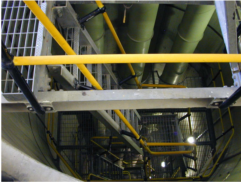
Figure 1.2: Mounting of the Drakensberg Pump Storage Station 400 kV GIL in vertical shaft, used with permission
