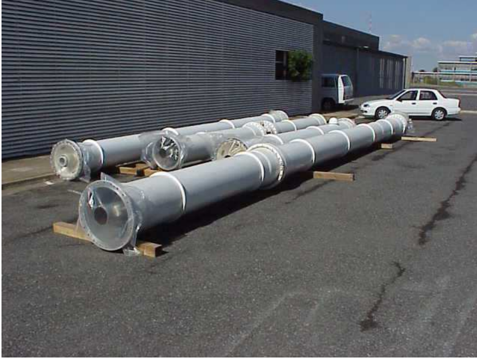
Figure 1.6: GIL on site, prior to installation, used with permission
