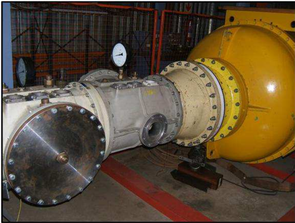
Figure 5.2: 750 kV transformer and duct setup
