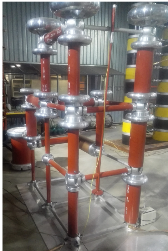
FIGURE 4.6: 400 kV DC Generator at WITS
