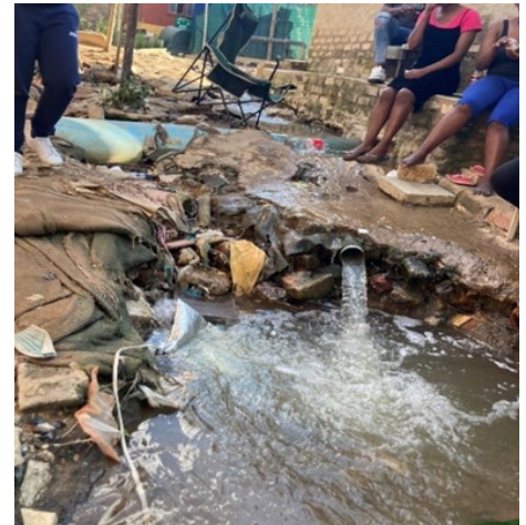
Figure 5.10 Makeshift drainage system built by the community (Source: Hopa, Kya Sands, 2022)
