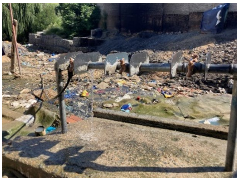
Figure 5.3: Leaking standpipes (Source: Hopa, Kya Sands, 2022)
