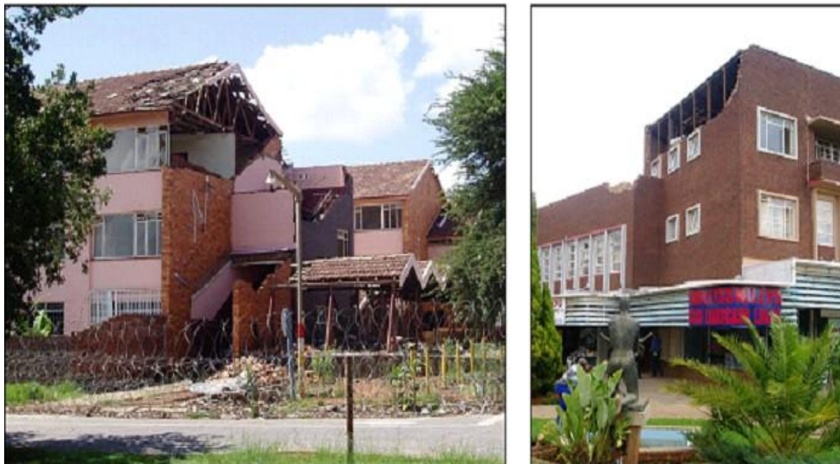
Figure 3.4: Damaged buildings at in Stilfontein resulting from an M_L 5.5 earthquake on 9 March 2005 (Durrheim et.al, 2014).
