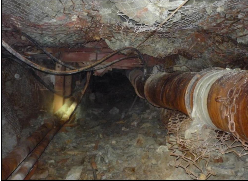
Figure 5.15: Damage to 38 cross-cut S showing unravelling of support including sidewall and hanging wall ejection of rock (Tshepo Rabele, 2014).
