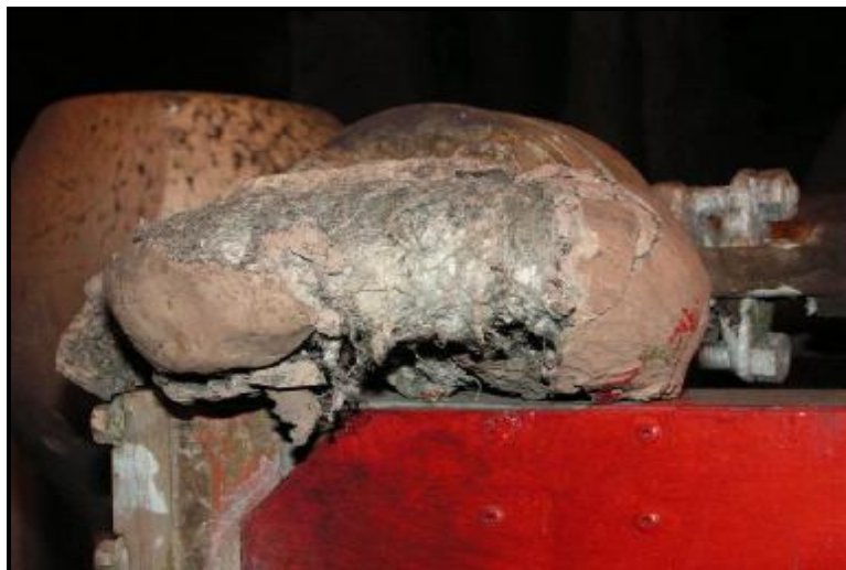
Figure 3.2: Removed hardset from pipe-work exposing asbestos insulating material beneath
