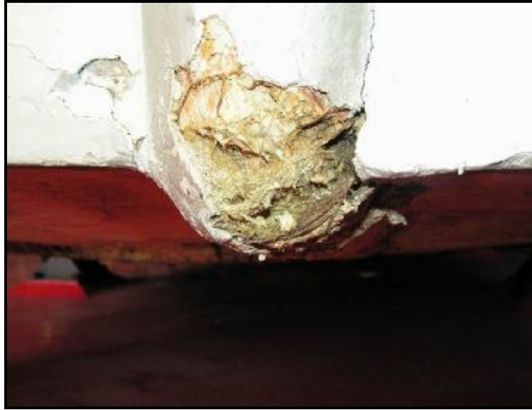
Figure 3.1: Removed hardset from a boiler's outer casing exposing asbestos insulating material beneath
