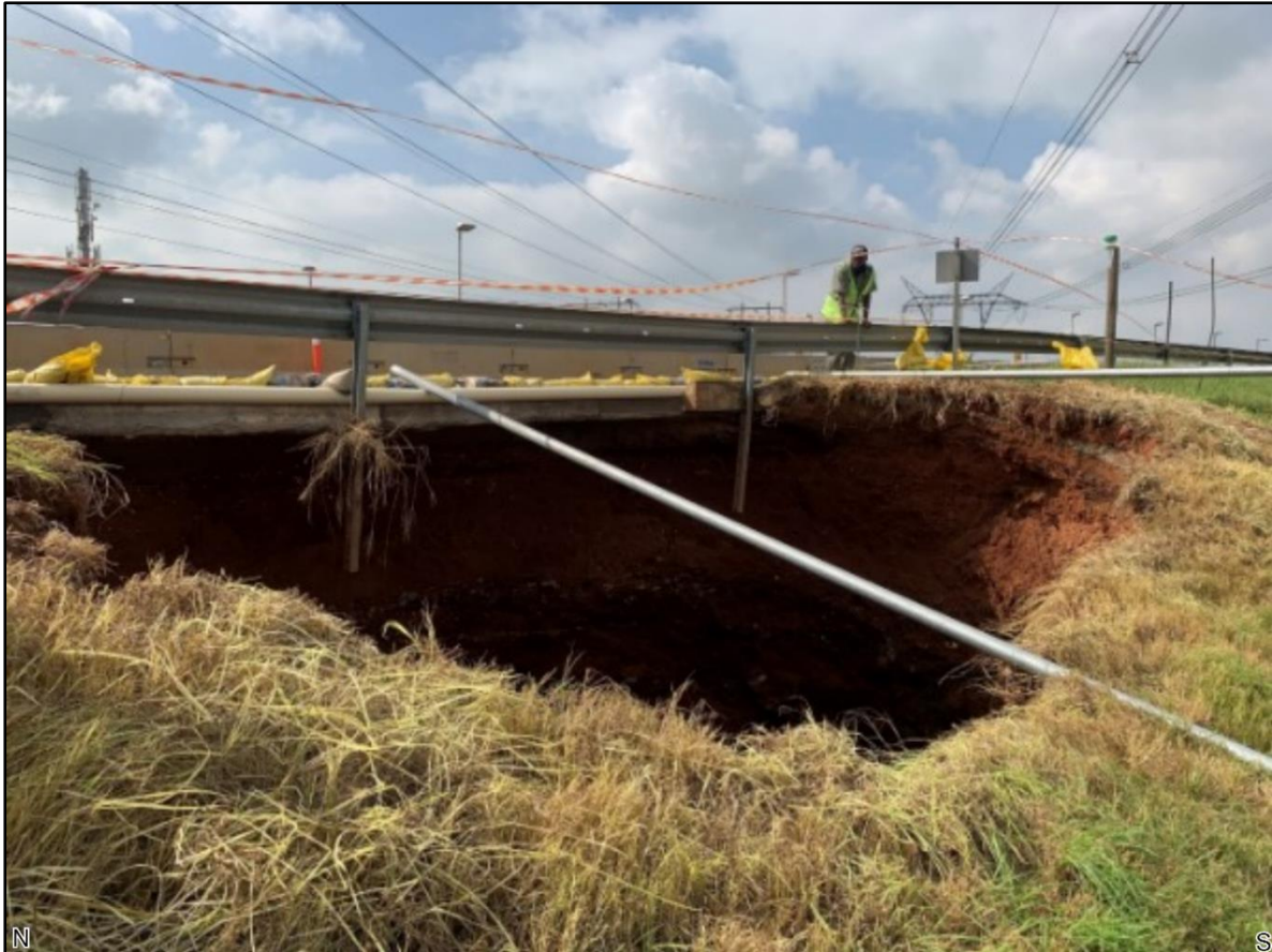
Figure 1.2: Image of a sinkhole that had formed on the R21 highway, in South Africa (Mabele, 2022).
