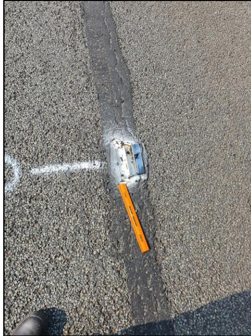
Figure 7.7: Metal pieces found on the R21 highway, which could have caused noise on the data.
