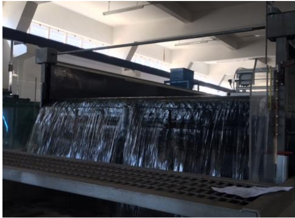
Figure 3-5: Water flowing over sluice gate
