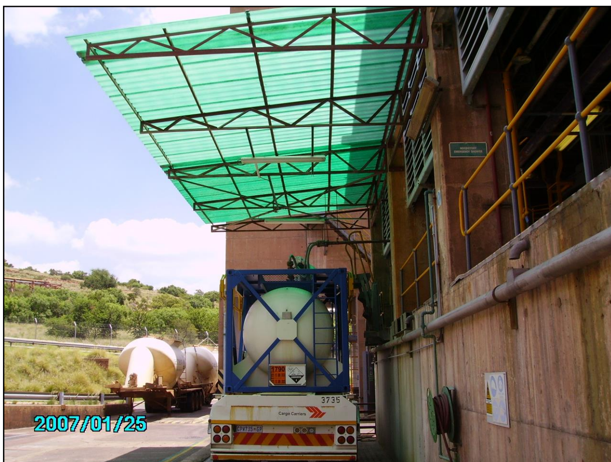
Figure 2.5: HF storage tank loading and transportation facility located on site at Necsa.
