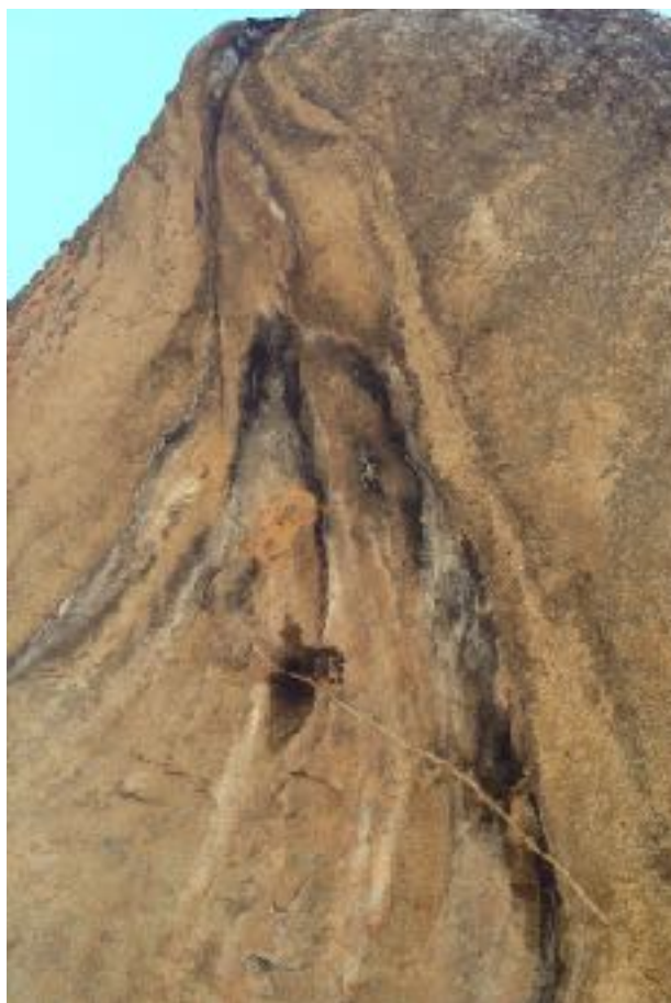
Fig. 5.19: A deep line etched into the upper region of the boulder presumably to redirect water away from the paintings (2016 digital colour photographs by L. de Harde).
