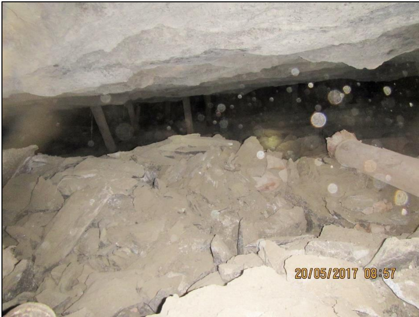
Figure 33: Footwall heave around the failed Merensky Reef pillar
