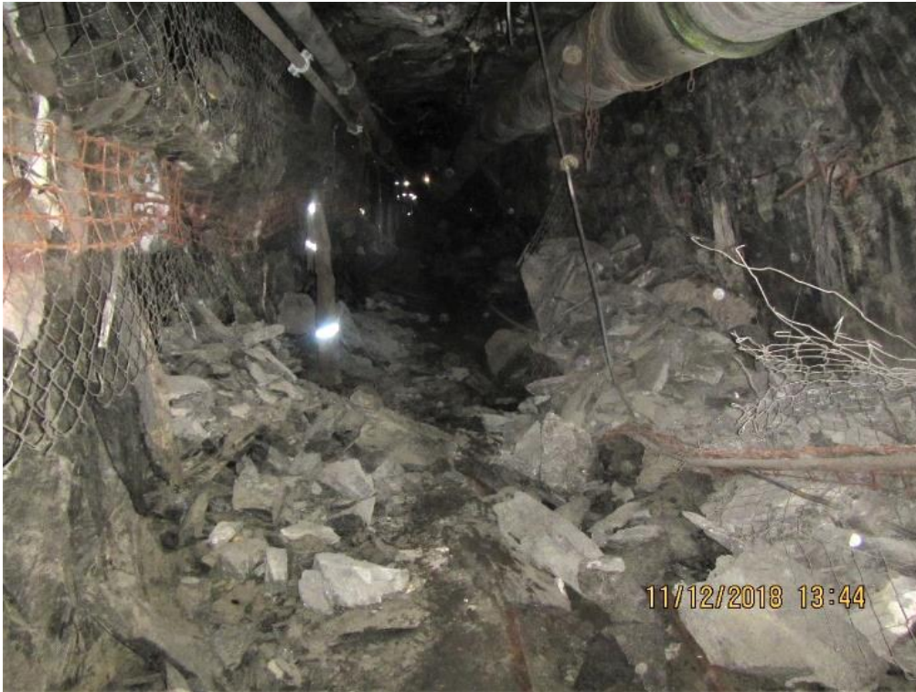
Figure 16: Photograph showing the 14-23W crosscut after dynamic failure
