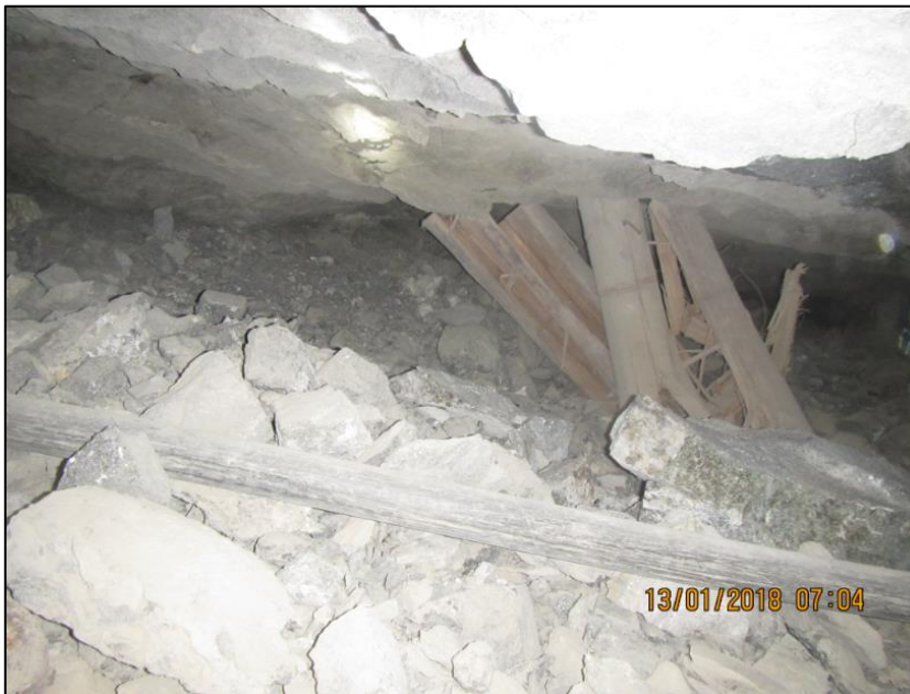
Figure 50: The footwall heave around the failed Merensky Reef pillar
