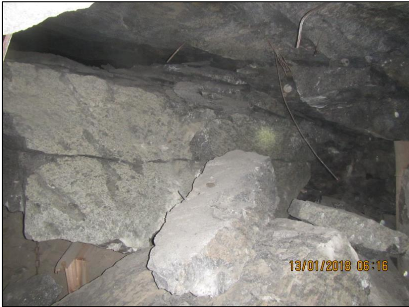
Figure 46: Hangingwall detachment of the Merensky Reef hangingwall
