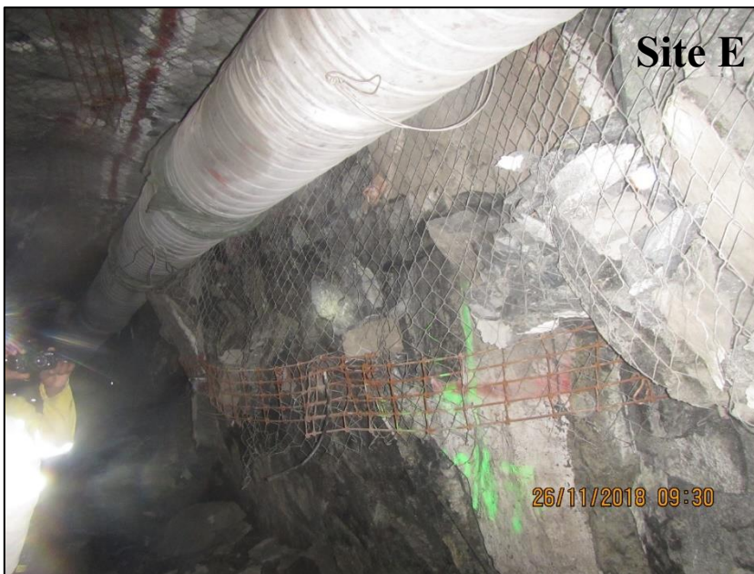
Figure 77: 14-23W UG2 crosscut - western sidewall. The secondary support in this area was highly tensioned as the cable anchors were observed to be pulled into the sidewall. This sidewall was very unstable
