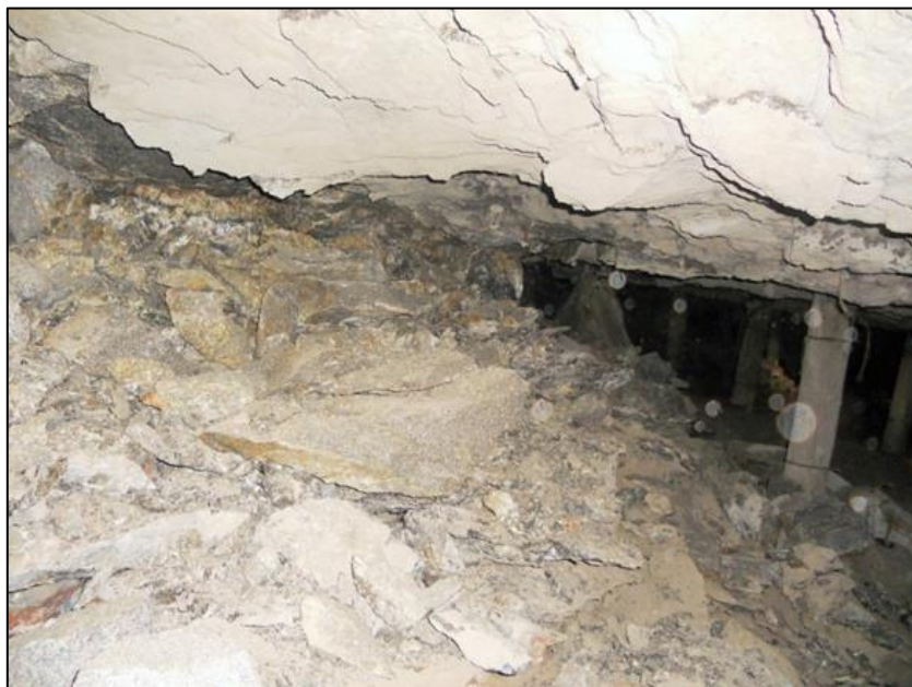
Figure 39: Damage to Merensky Reef pillar
