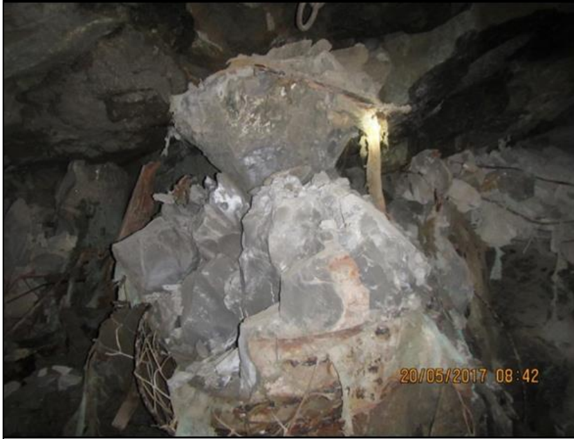
Figure 28: Grout pack failure showing excessive closure. These grout packs were adjacent to the centre gully. This pack was originally 1.0 m in diameter
