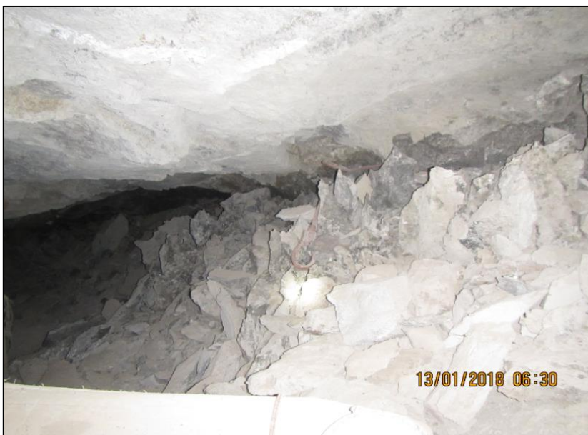
Figure 49: Crushed (completely failed) Merensky Reef pillars
