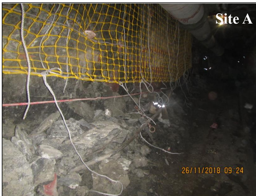
Figure 73: 14-23W UG2 crosscut - western sidewall - Approximately 20 m from travelling way. Shake-down damage. This sidewall was previously reported to be scaling excessively. Net was installed as a remedial measure
