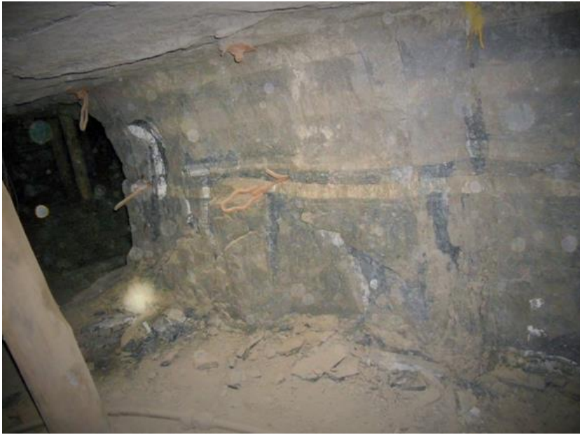
Figure 42: Damage to the superimposed UG2 Reef pillar
