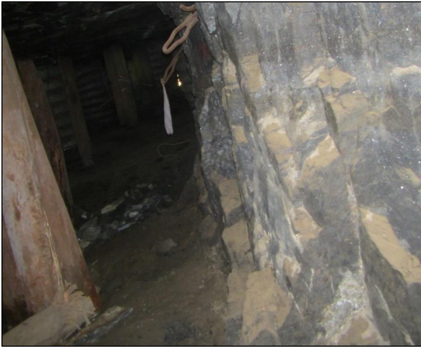
Figure 36: The superimposed UG2 Reef pillar corner, which had little sign of damage
