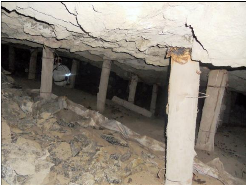
Figure 41: Footwall heave around the failed pillar
