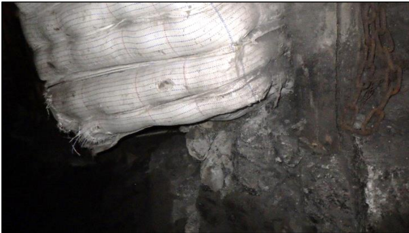
Figure 85: Damaged pack in centre gully showing the footwall failure below the grout pack
