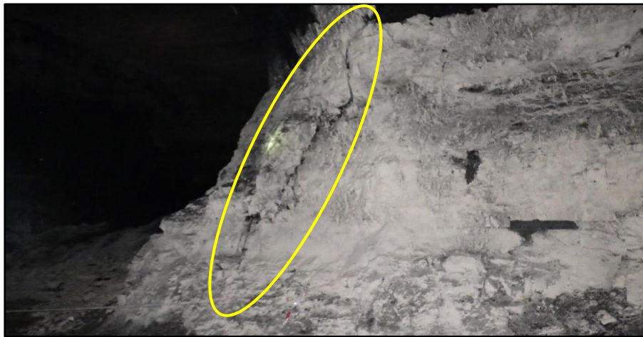
Figure 3.2-3-Observed slip failure along pillar rib at No.2 Seam, Goedehoop colliery ( AngloAmerican (Thermal coal), 2017 )
