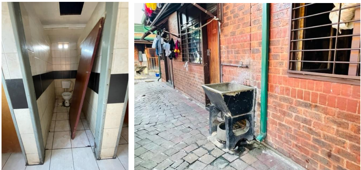
(Figure 4.5b) Services at Kwa Mai Mai. (Author's own). The images above show the water and sanitation services available at the market. Evidently, these were designed to serve the traders and customers at the market during the day. The deteriorated conditions can be notes specifically in the toilet area which still requires a payment of R2 with every use.
