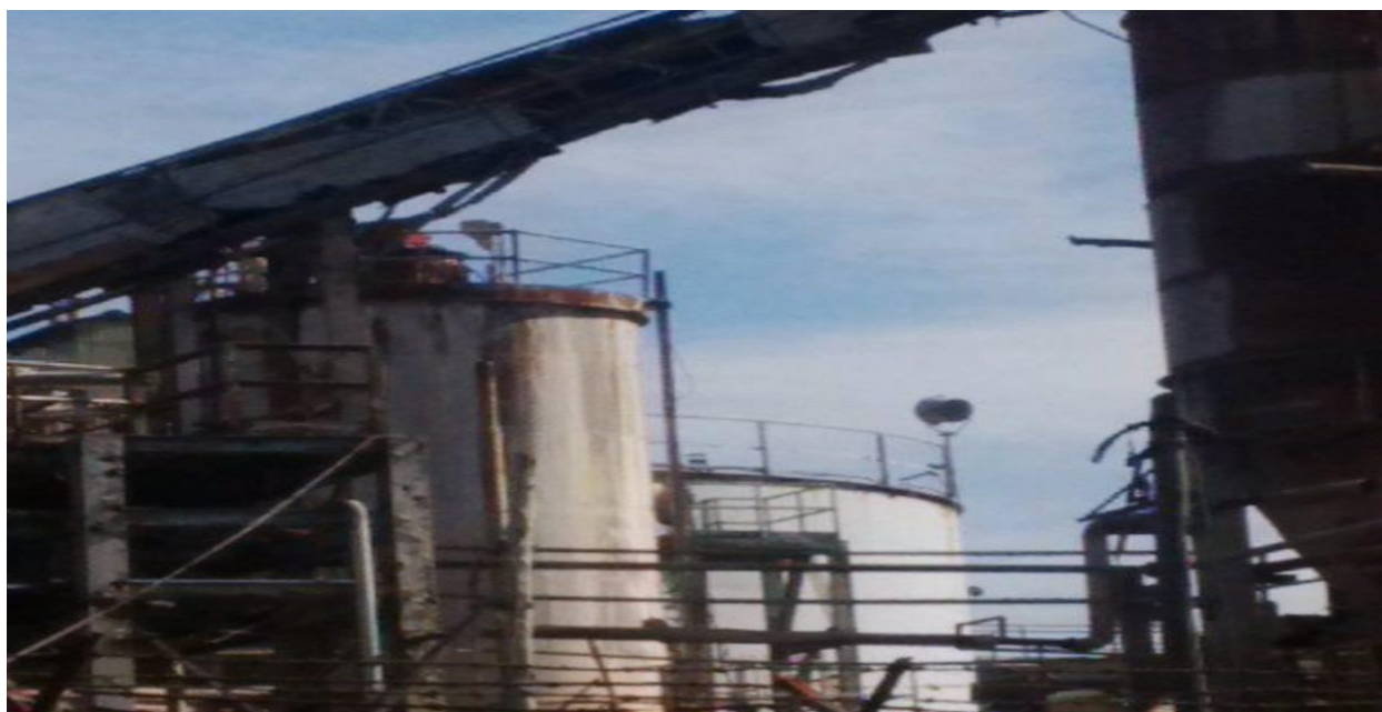
Fig. 15: Photo courtesy of internet, (2021) showing the dilapidated Webuye Paper Mill in Webuye town, Webuye West constituency, Bungoma County.
