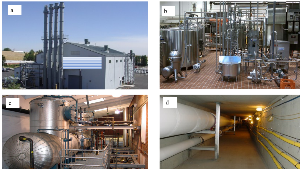
Figure 4.2: The case study of a manufacturing factory investigated in this study. Note: a) front view of the manufacturing plant; b) the evaporation processing unit; c) the steam boilers used mainly in the heating/pasteurization unit; d) the steam network to other processing units.
