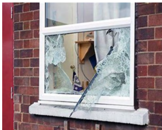
Picture 4.4: Showing a broken window (an indicator of burglary)
