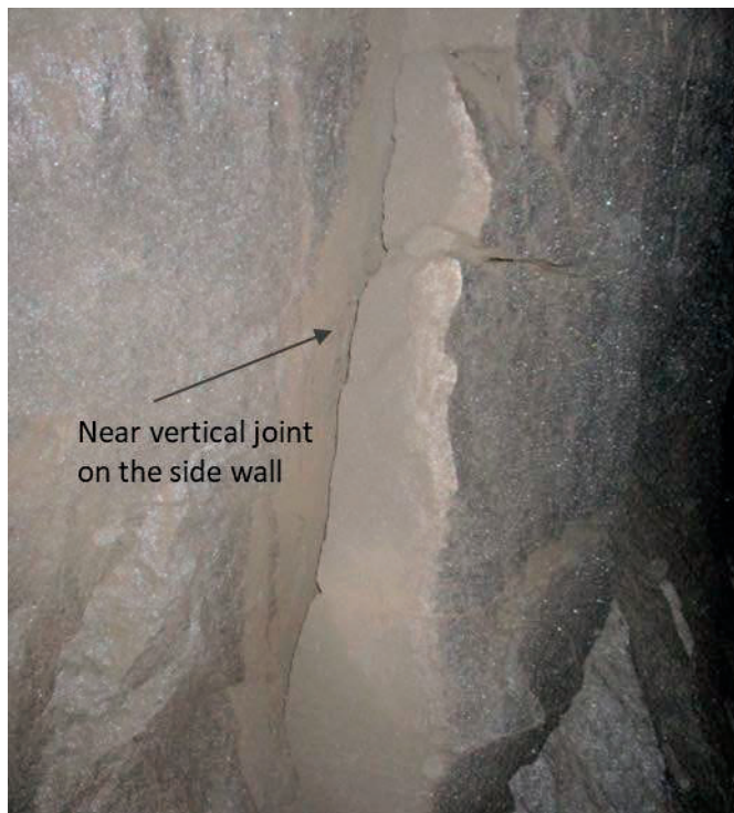
Figure 6.1: Near vertical joint on side wall (LG6 seam)
