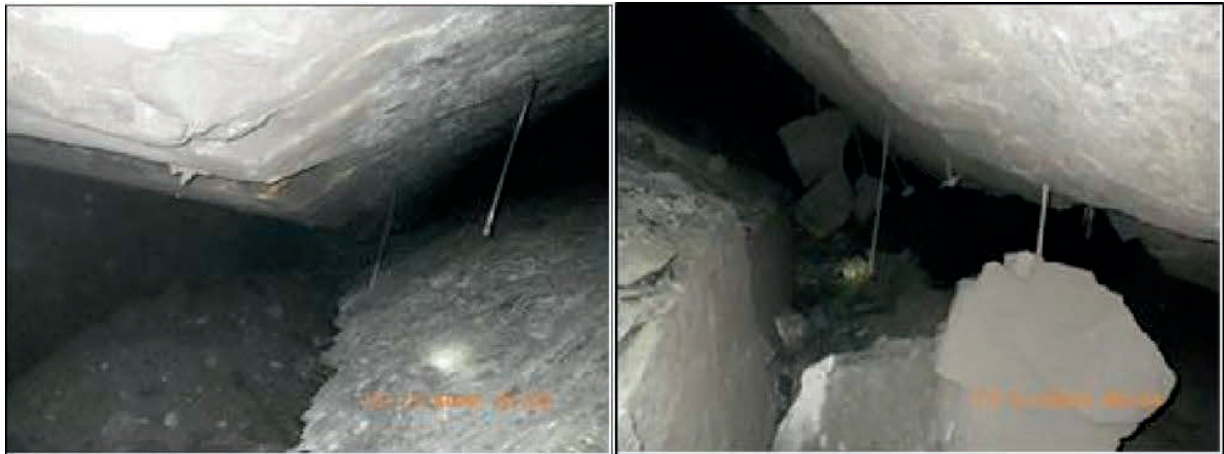
Figure 2.8: Wedge failure (Qamata & Steenkamp, nd)
