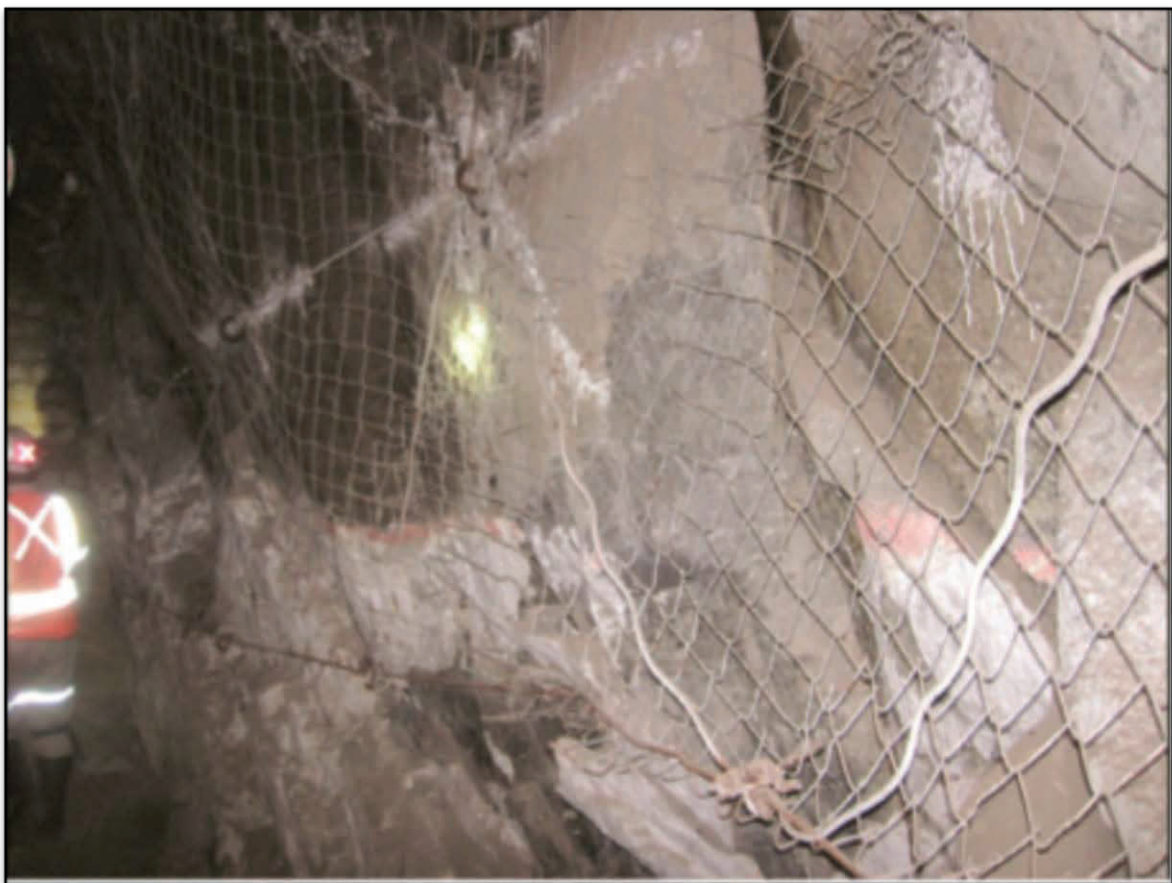
Figure 2.9: Spalling in a haulage tunnel in a platinum mine located in the western Limb of the BC (Nyungu & Stacey, 2014)
