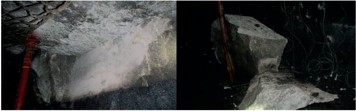
Figure 4.5: Wedge failure at the face area (Internal Mine Document, 2018)
