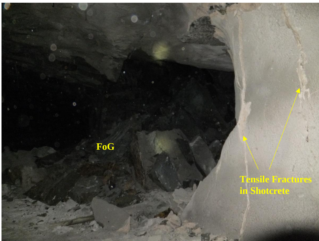
Figure 15: Shotcrete failure against the sidewalls
