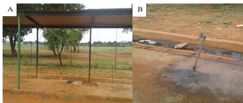
Figure 25: Standpipes in front of Carousel Hotel (A & B)
