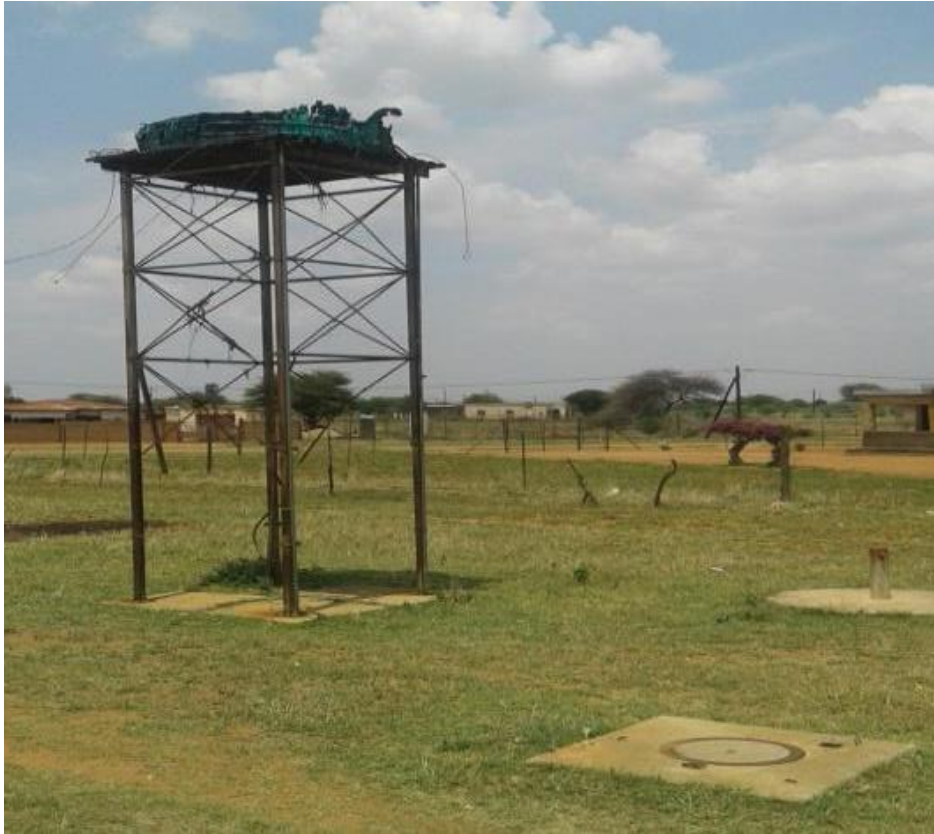
Figure 22: Burned public water tank as a result of the water protests
