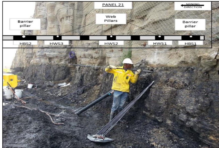
Figure 5-5: Installation of the sensors and relative positions in panel 21
