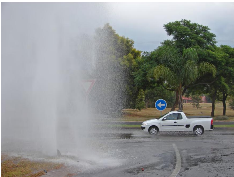
Figure 5: Physical Leakage Due to Pipe Failure, (Mckenzie et al., 2012)
