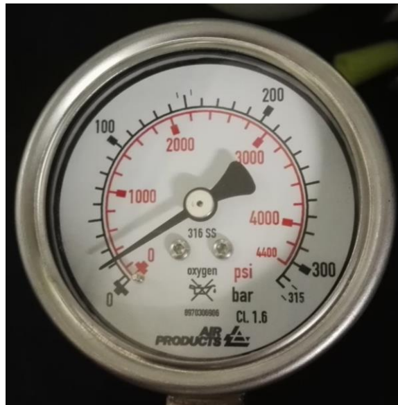
Figure 4-20 : Calibration of regulator pressure gauge
