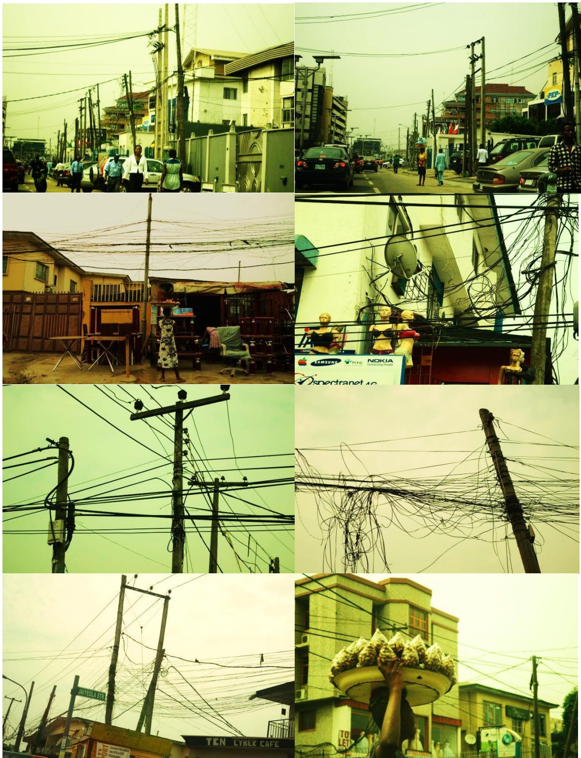
Figure 27: The criss-crossing electricity power lines in Lagos.
