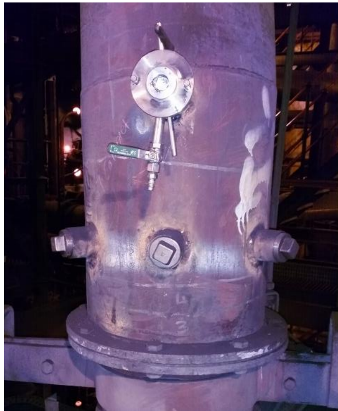
Figure 3-4: Sampling Ports at Pipe P1
