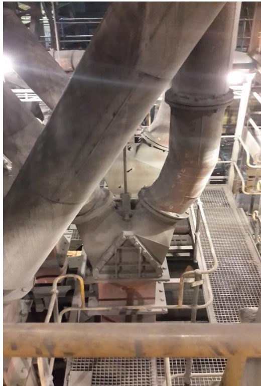
Figure 4-9: PF Pipes P1 & P2 Exiting Riffle Box
