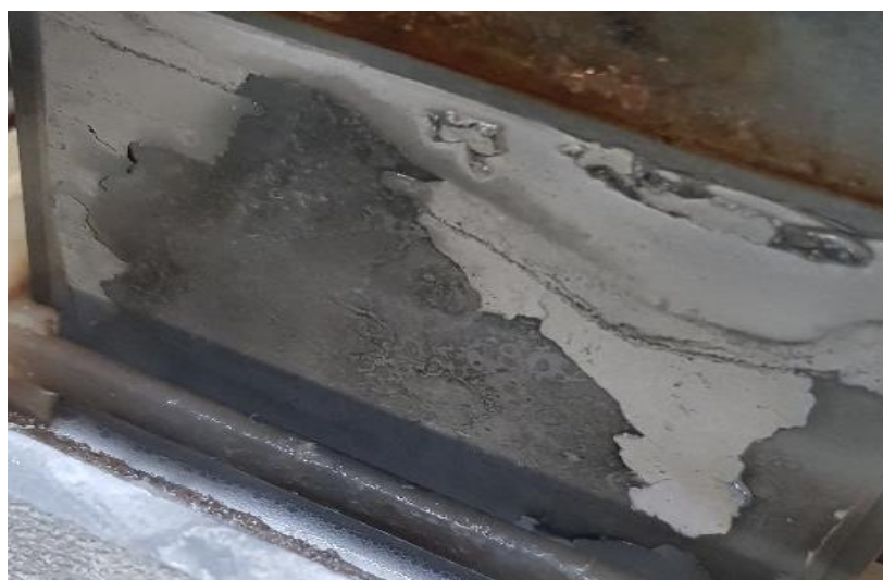
Figure C.4 Deposit flaking from the second cathode of trial 2
