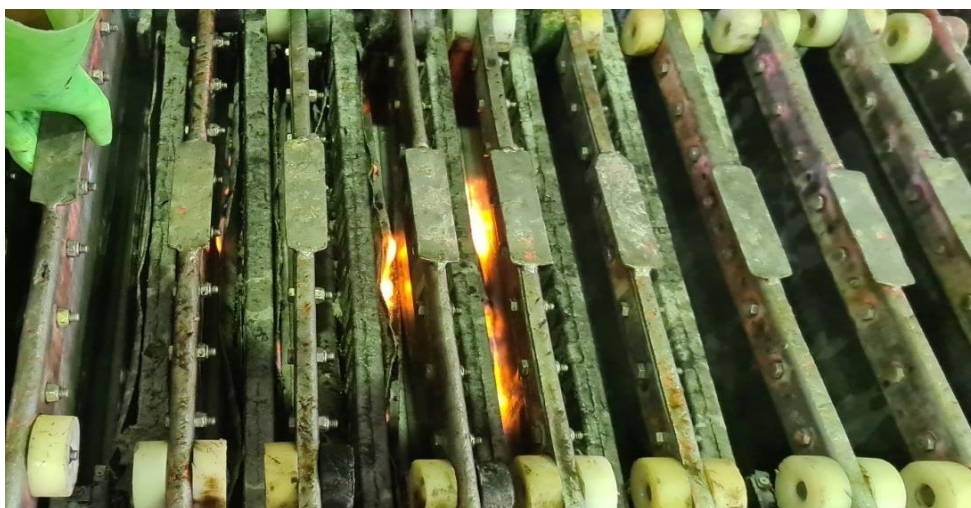
Figure D.10 Hydrogen fire occurring in the cellhouse mostly when there is water leak in the cellhouse or during the cracking and flaking condition of the cellhouse
