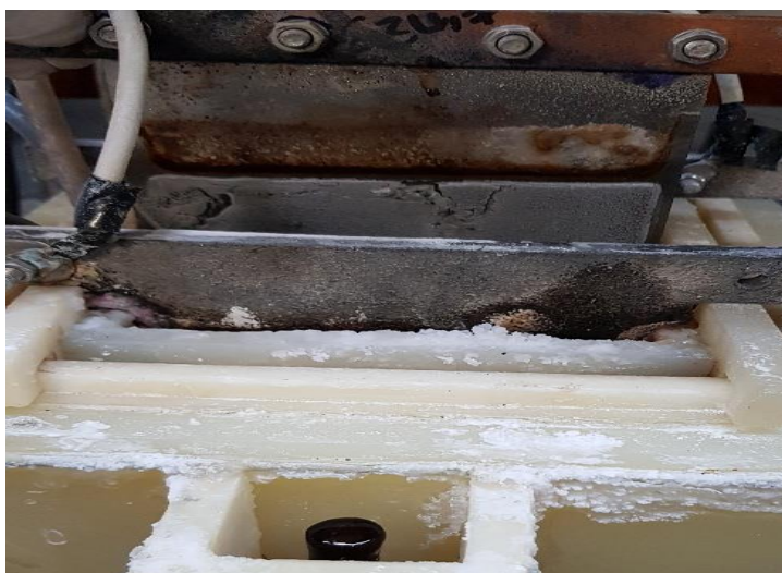
Figure D.8 Observation of cracking at the of top part of cathode plate during run 4
