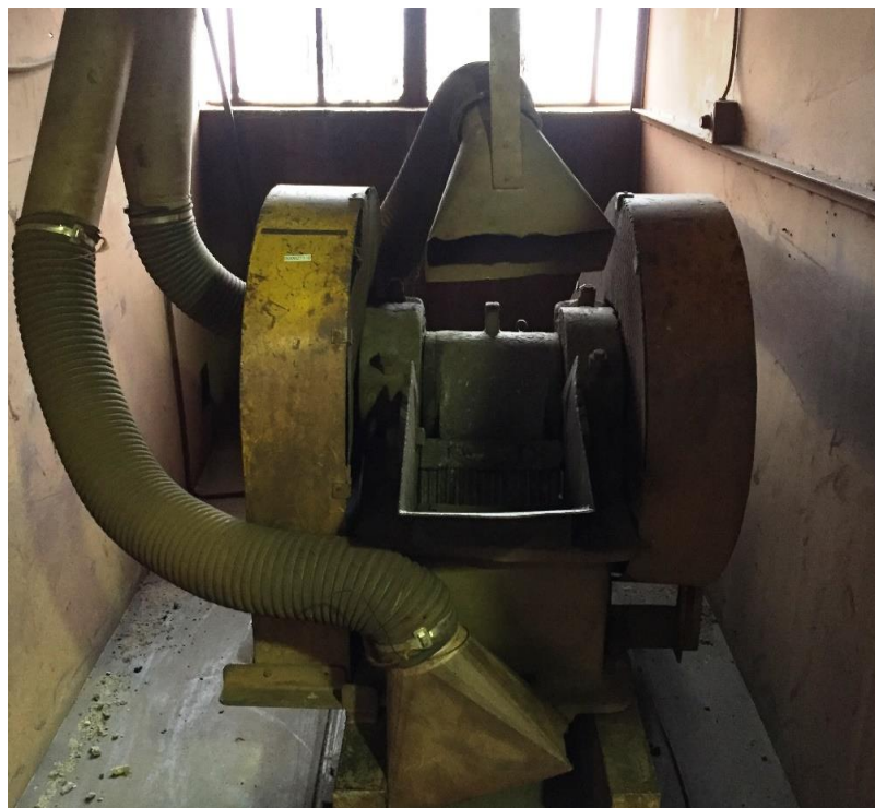
Figure 6 – Cone Crusher (Exxaro)
