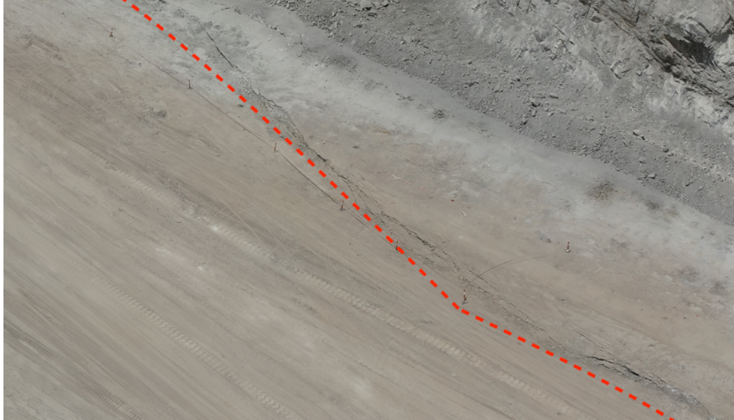
Figure 4-8: Large cracks were observed in Phase Three (Aero Vision Drone Services, 2022).
