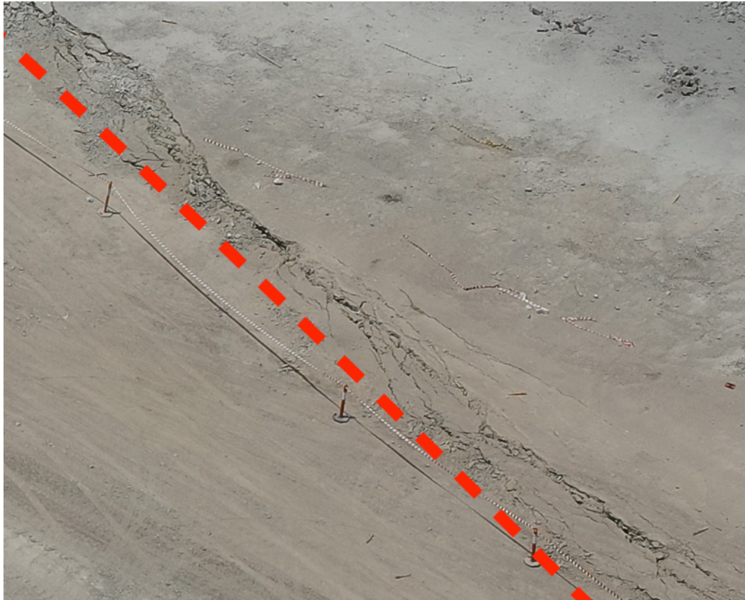
Figure 4-9: A zoomed-in image of the cracks observed in Phase Three (Aero Vision Drone Services, 2022).
