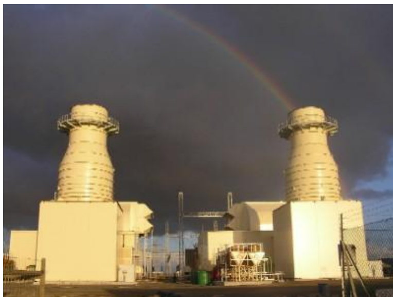
Figure 33 - Ankerlig Open Cycle Gas Turbine Plant
