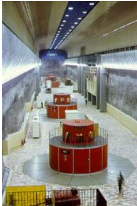
Figure 35 - Drakensburg Pump/Turbine Hall
