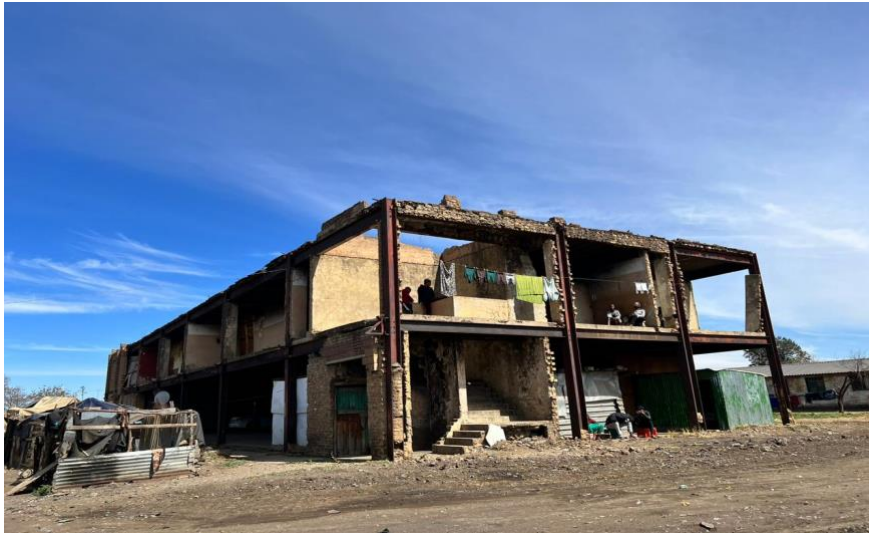
Image 1: A dilapidated shopping centre abolished post-democracy located at Mshayazafe Hostel, Thokoza
