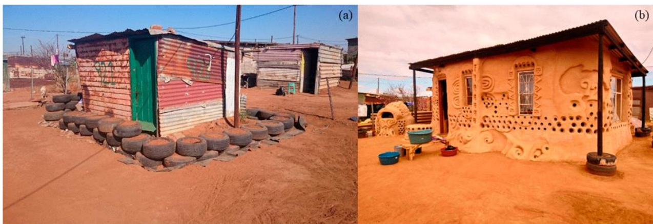
Figure 2: An earthship house under construction by one of five participants in Venter , et al.’ (2019) study.
