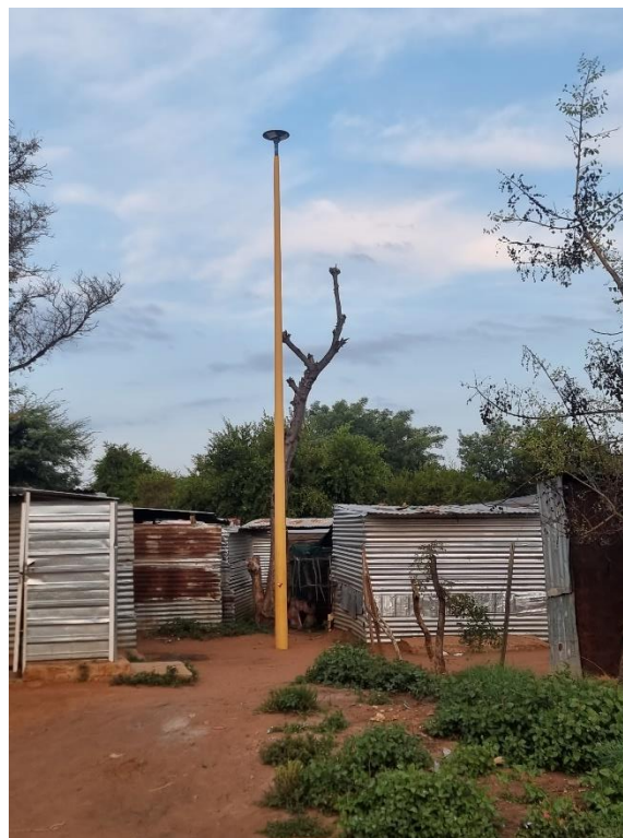
Figure 10: Solar powered area lighting for crime prevention
