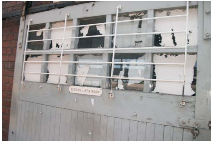
3.29. a dilapidated door
