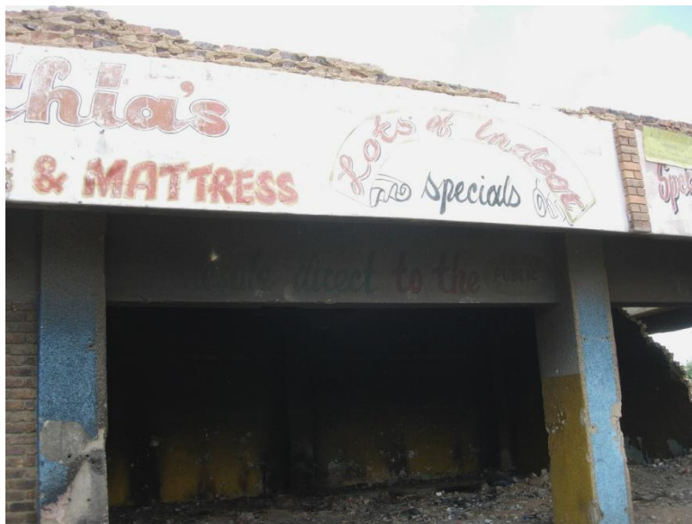
Figure 16 (2008): Burnt-out shops, once part of Kliptown's extensive commercial district. Photo: Naomi Roux
