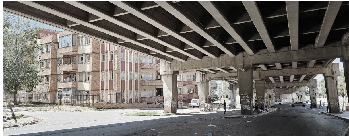
Figure 19: Highway underpass, under Joe Slovo Drive in Berea is a )transit anti- space (Author, 2024)
