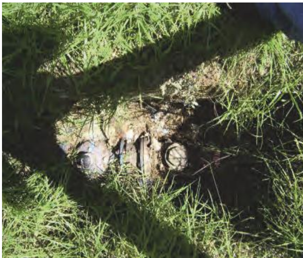
Figure 4.5: Meter buried in ground
