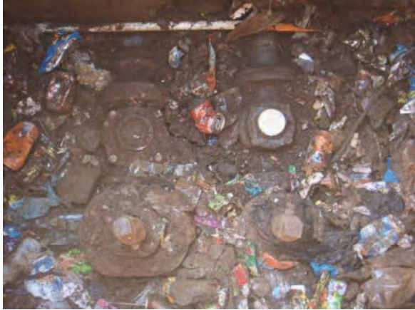
Figure 4.3: Buried and broken meters
