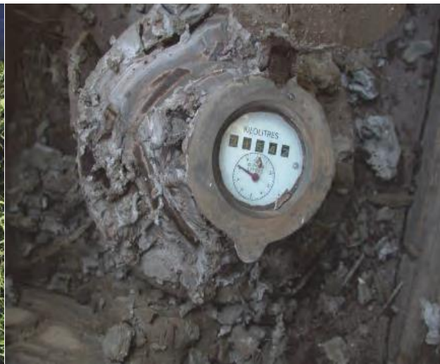
Figure 4.6: Non-functional and old meter
