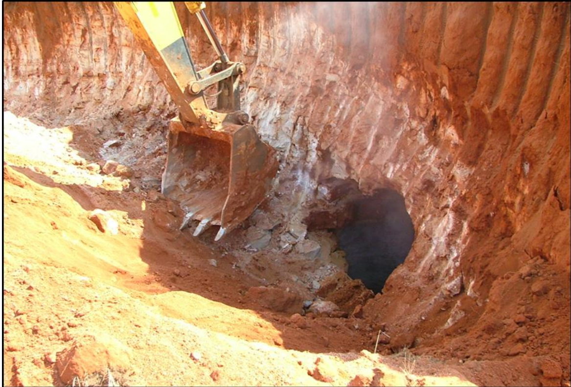
Figure 4-5: The Sinkhole exposure process
