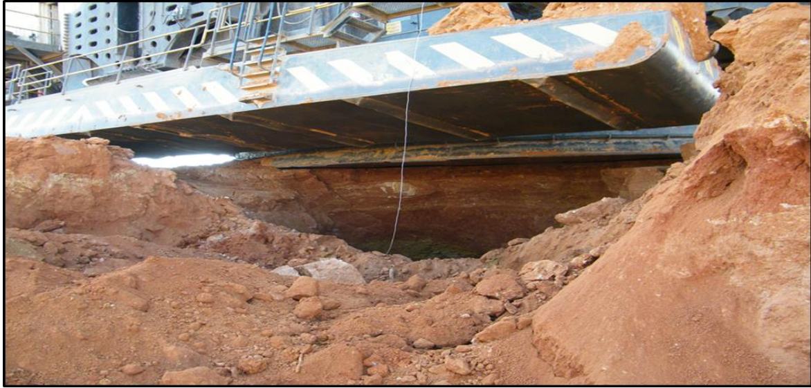
Figure 3-13: The dragline stuck in the residual sinkhole as indicated in the above picture.
