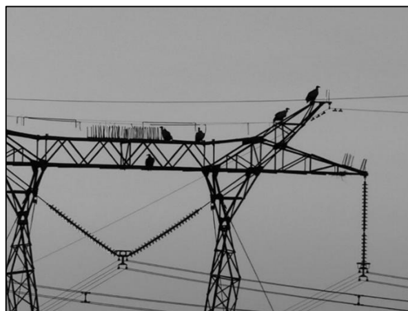
Figure 2-4: Cape Vultures roosting on an Eskom Transmission Power line, Eastern Cape by Kate Webster of CVC (2016).
